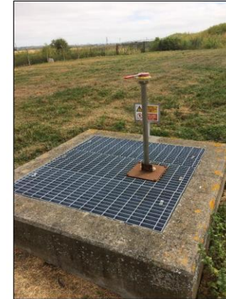
Figure 11: Gas condensate trap.
