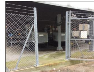
Figure 9: Gas booster compound.
