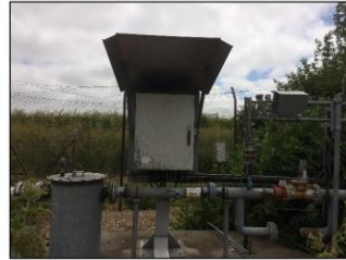
Figure 10: Flare stack compound.
