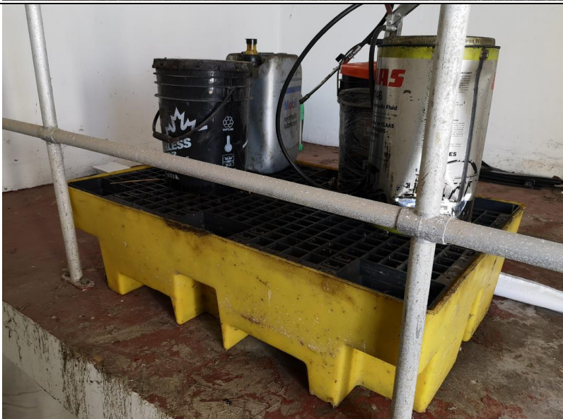
Bunding of chemicals
