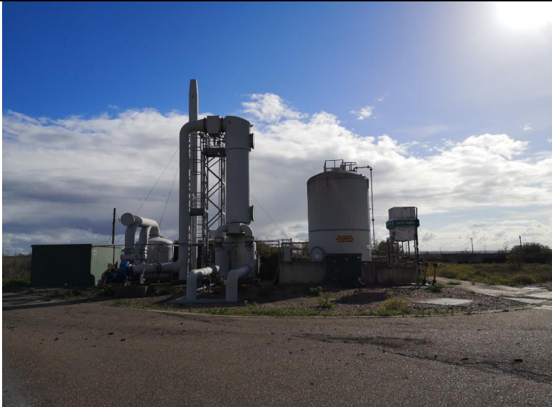
Odour unit - decommissioned
