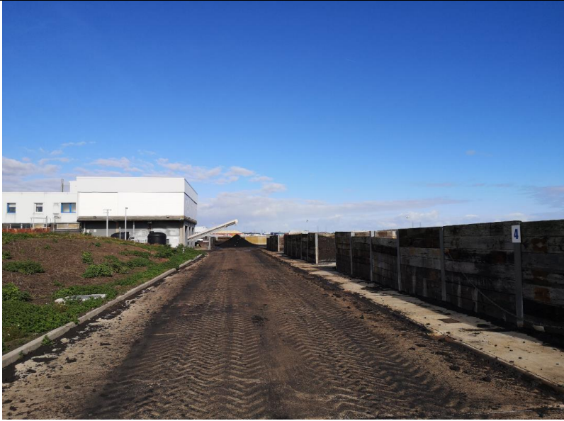
Road near cake bays in good condition although some tracking of cake
