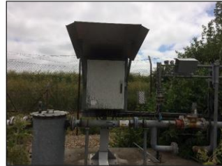
Figure 10: Flare stack compound.
