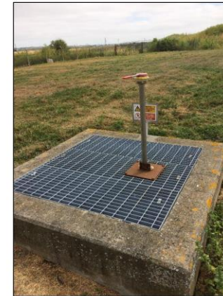
Figure 11: Gas condensate trap.
