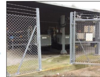
Figure 9: Gas booster compound.
