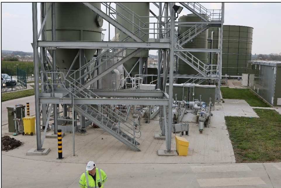
Figure 16. Centrate balance tank (background) with dosing tanks (foreground).
