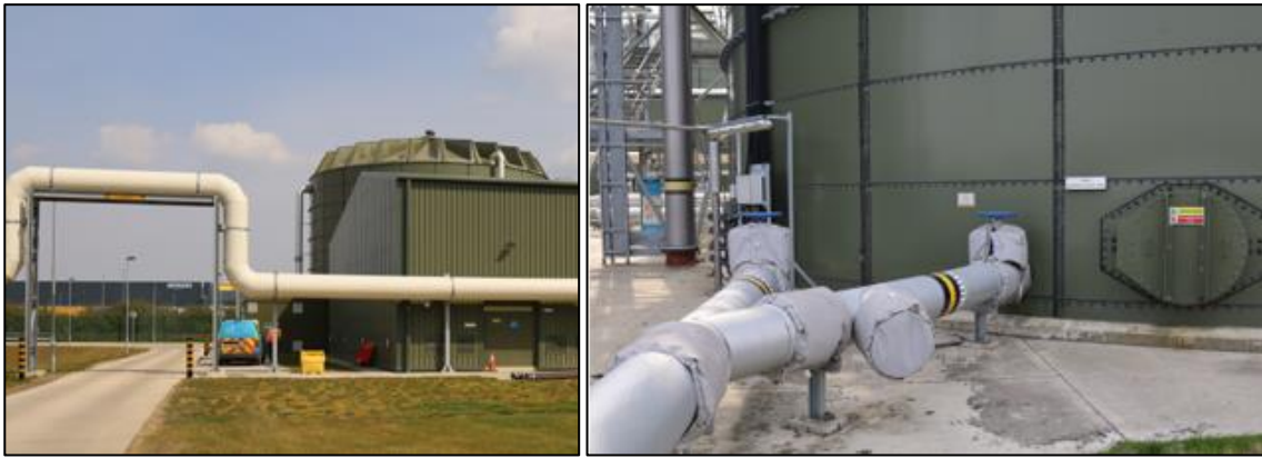
Figure 10. Left: screened sludge tank, right: pipe lagging.
