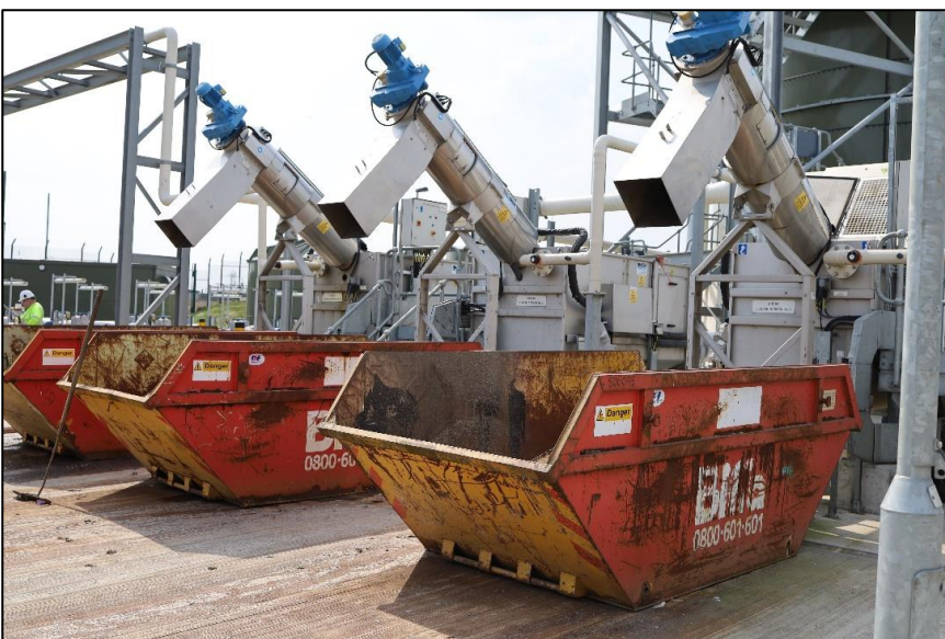
Figure 9. Enclosed rotating sludge screens and skips.
