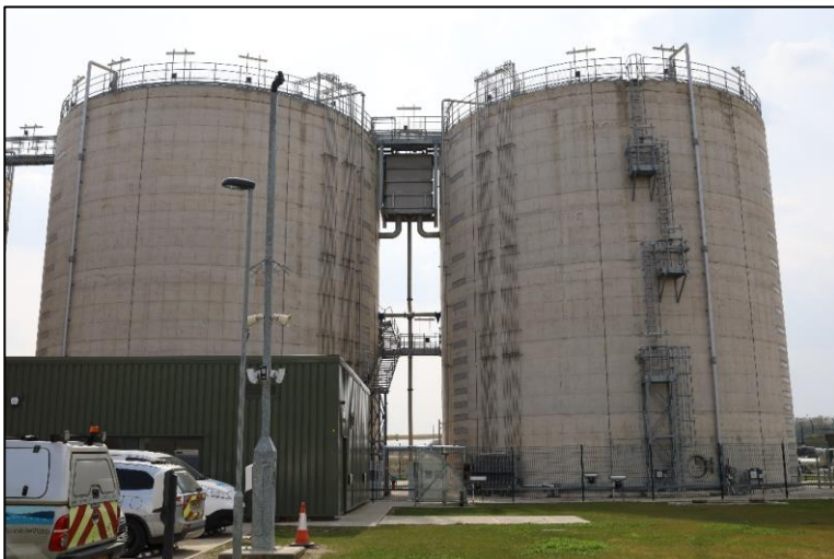
Figure 13. Two of four digester units.
