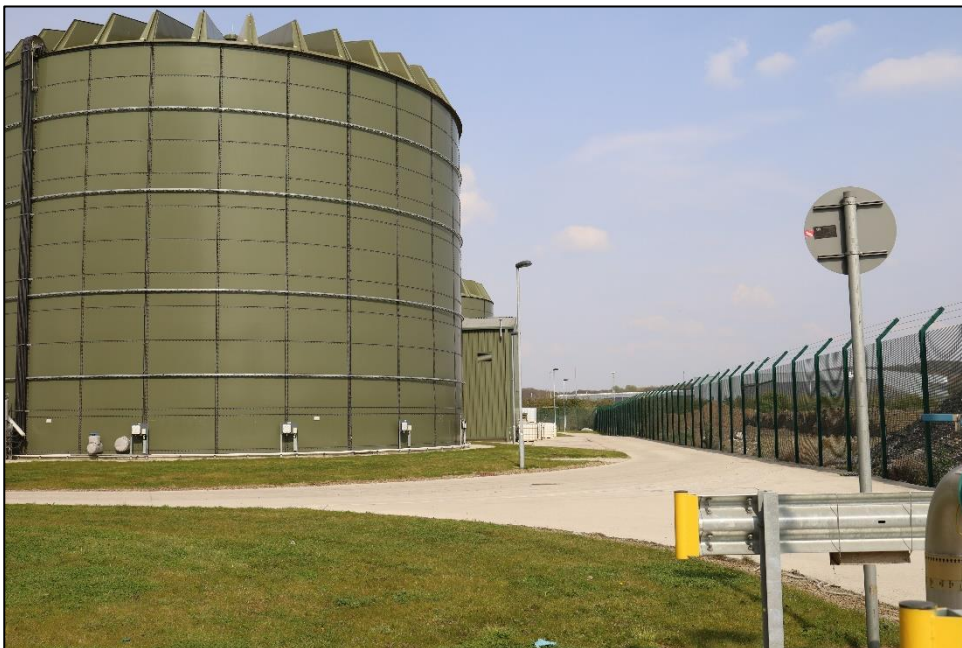
Figure 12. Digester feed tank.
