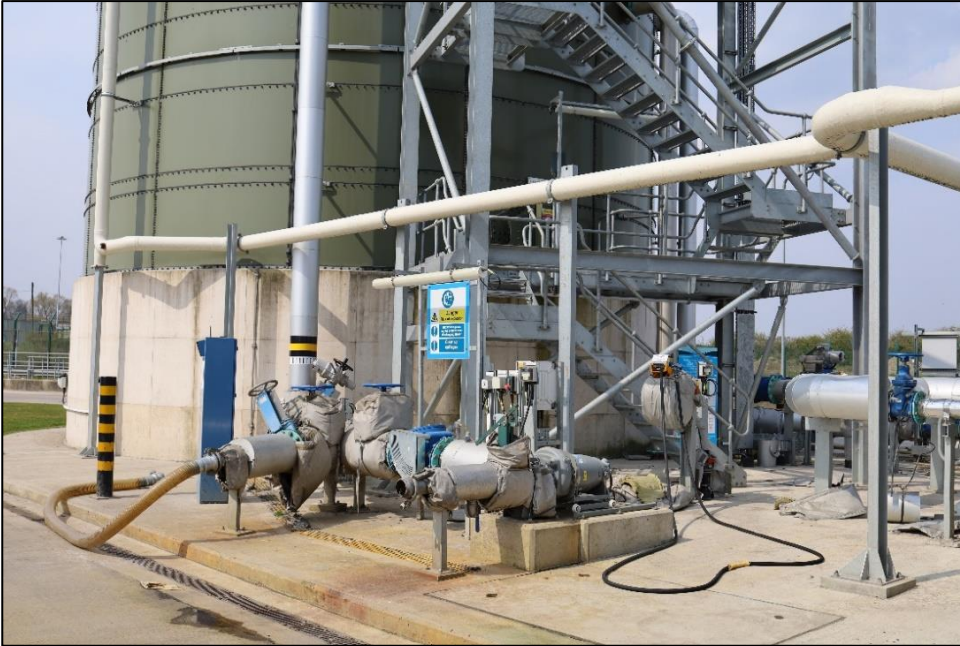
Figure 8. Sludge unloading area and sludge screen feed tank.
