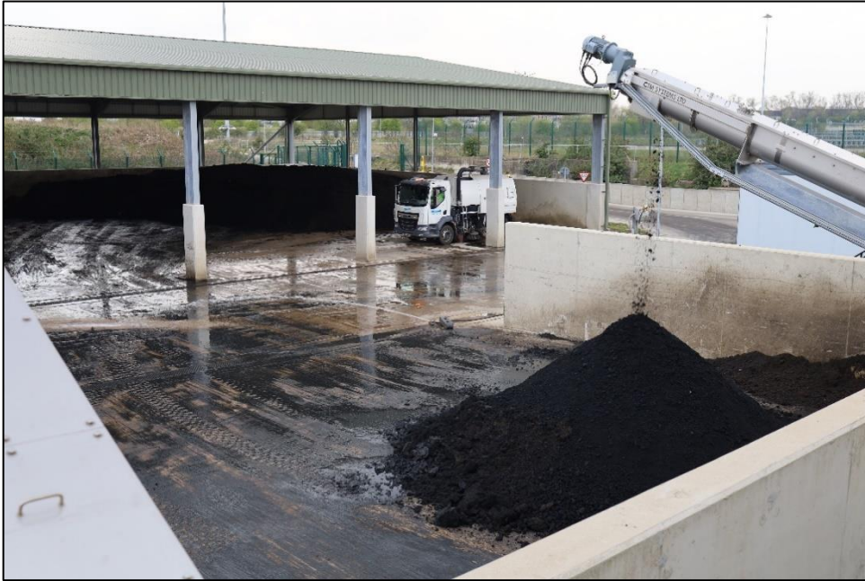
Figure 15. Digested sludge cake storage and loading pad.
