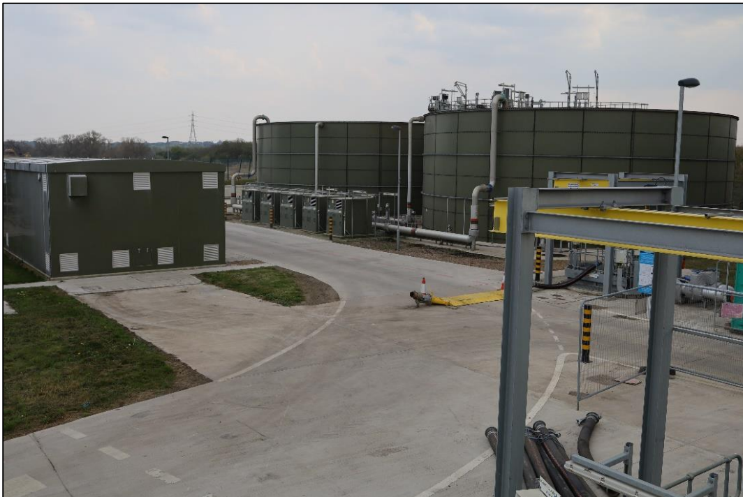
Figure 18. LTP reactor tanks.
