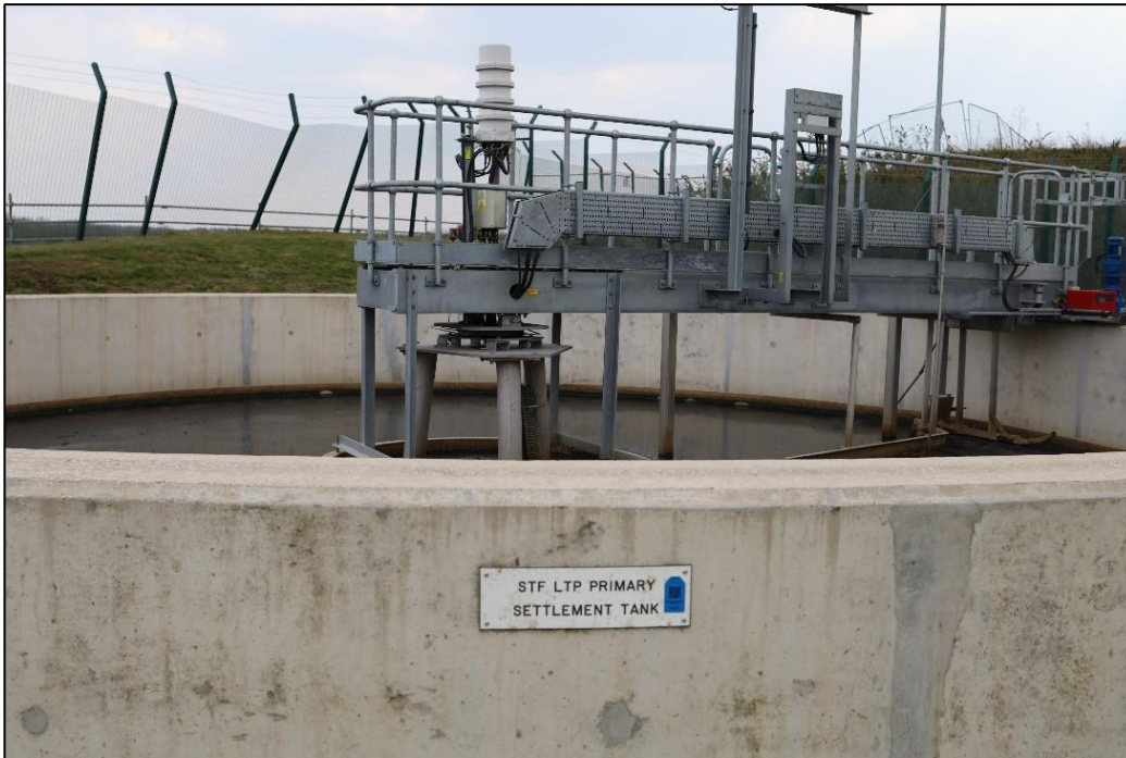
Figure 17. LTP primary settlement tank.
