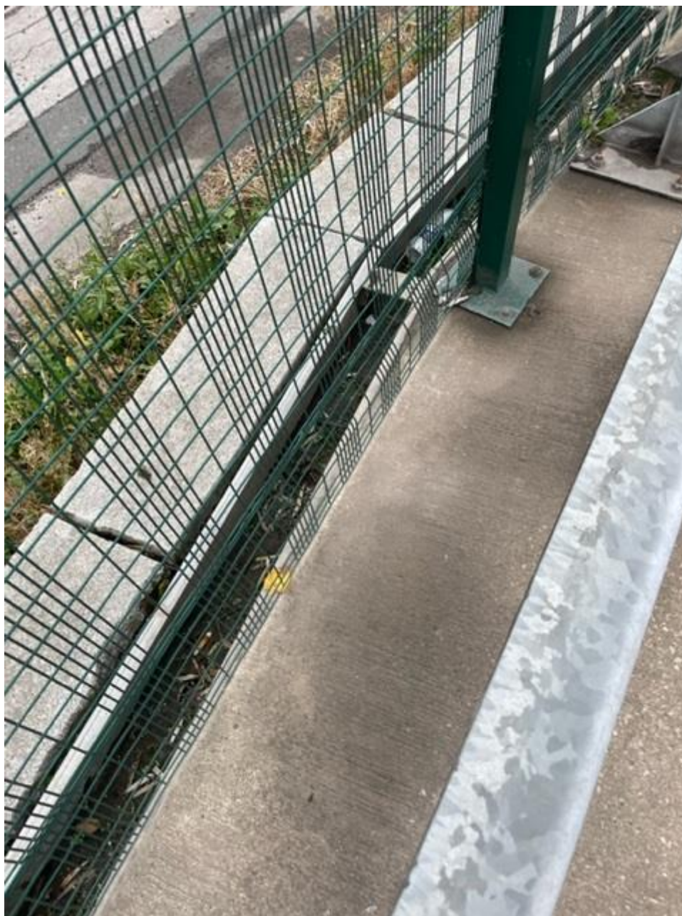
Car park drainage channels
