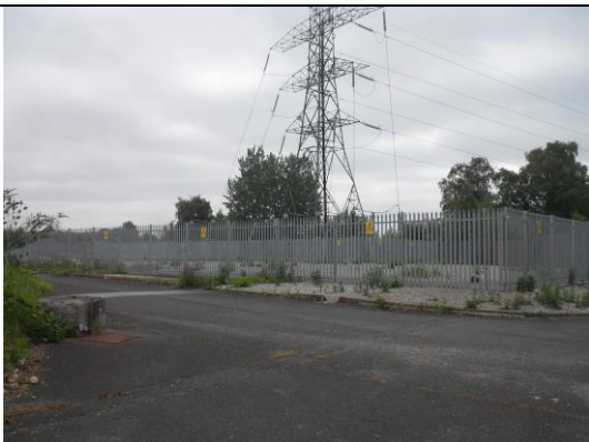
Transmission pylon compound (to remain)
