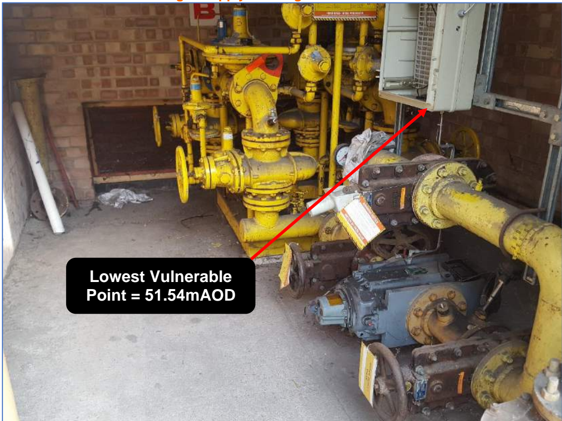
Photo 24 – Internal view of the gas supply building
