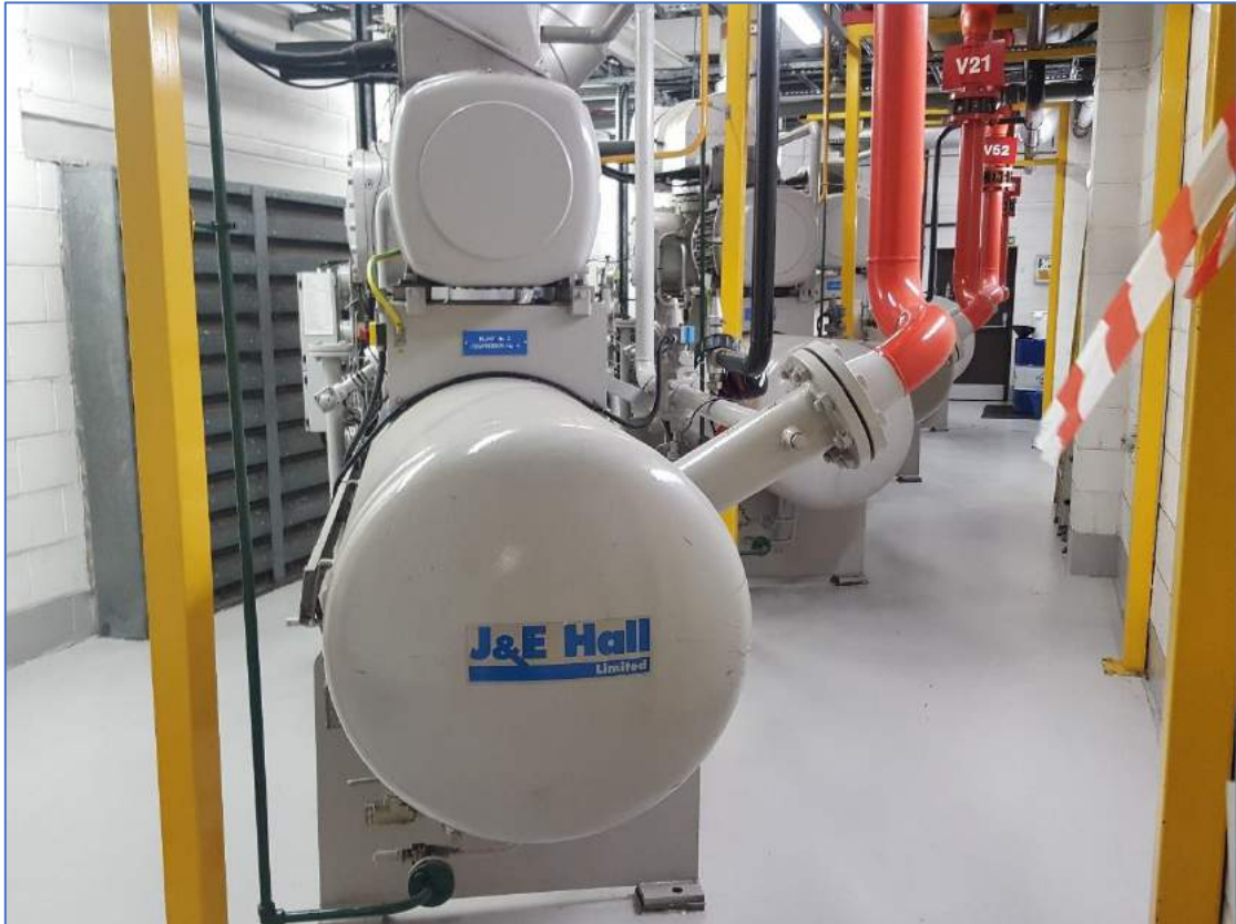
Photo 12 – Refrigeration plant in the production building
