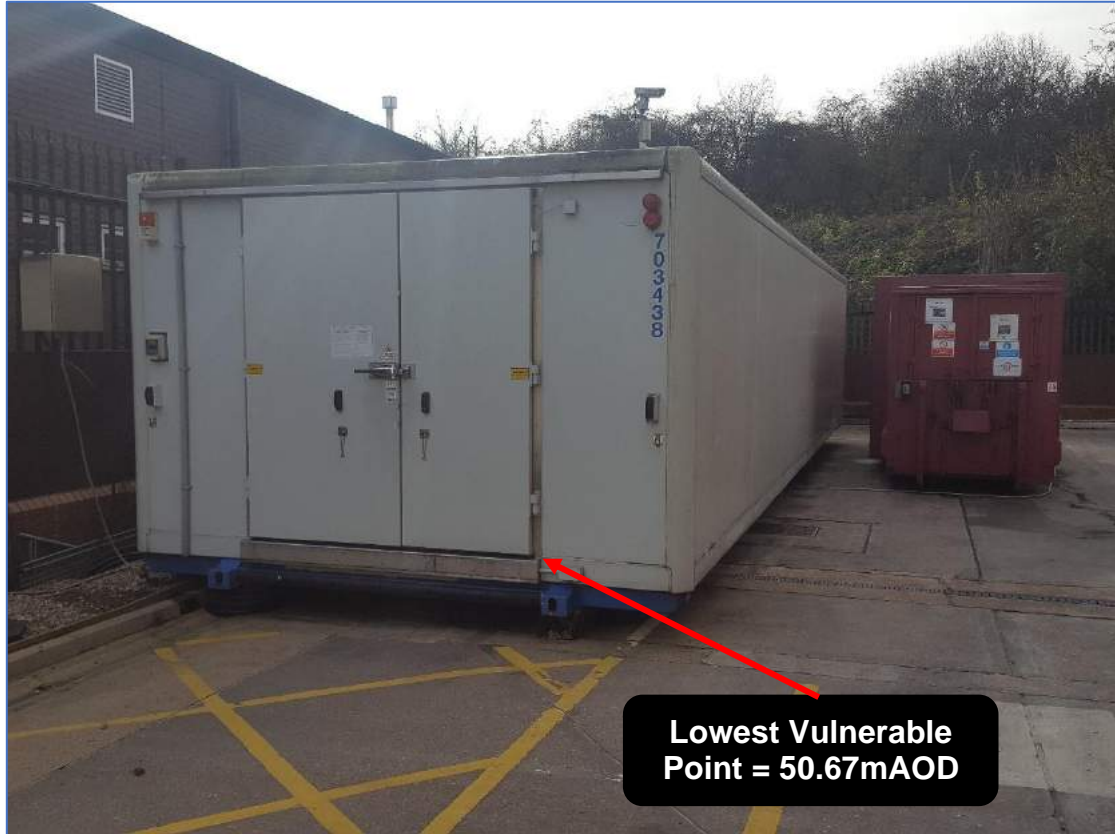
Photo 25 – External refrigeration container
