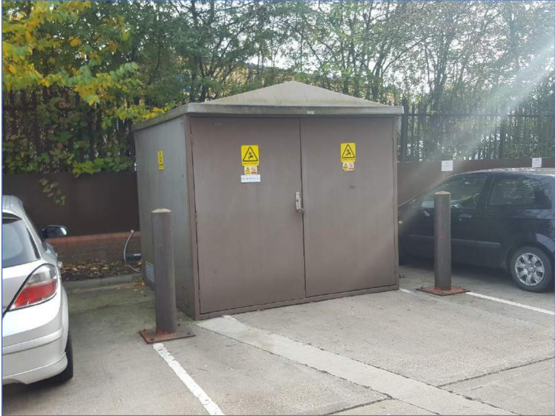
Photo 21 – Substation on the eastern perimeter of the production building
