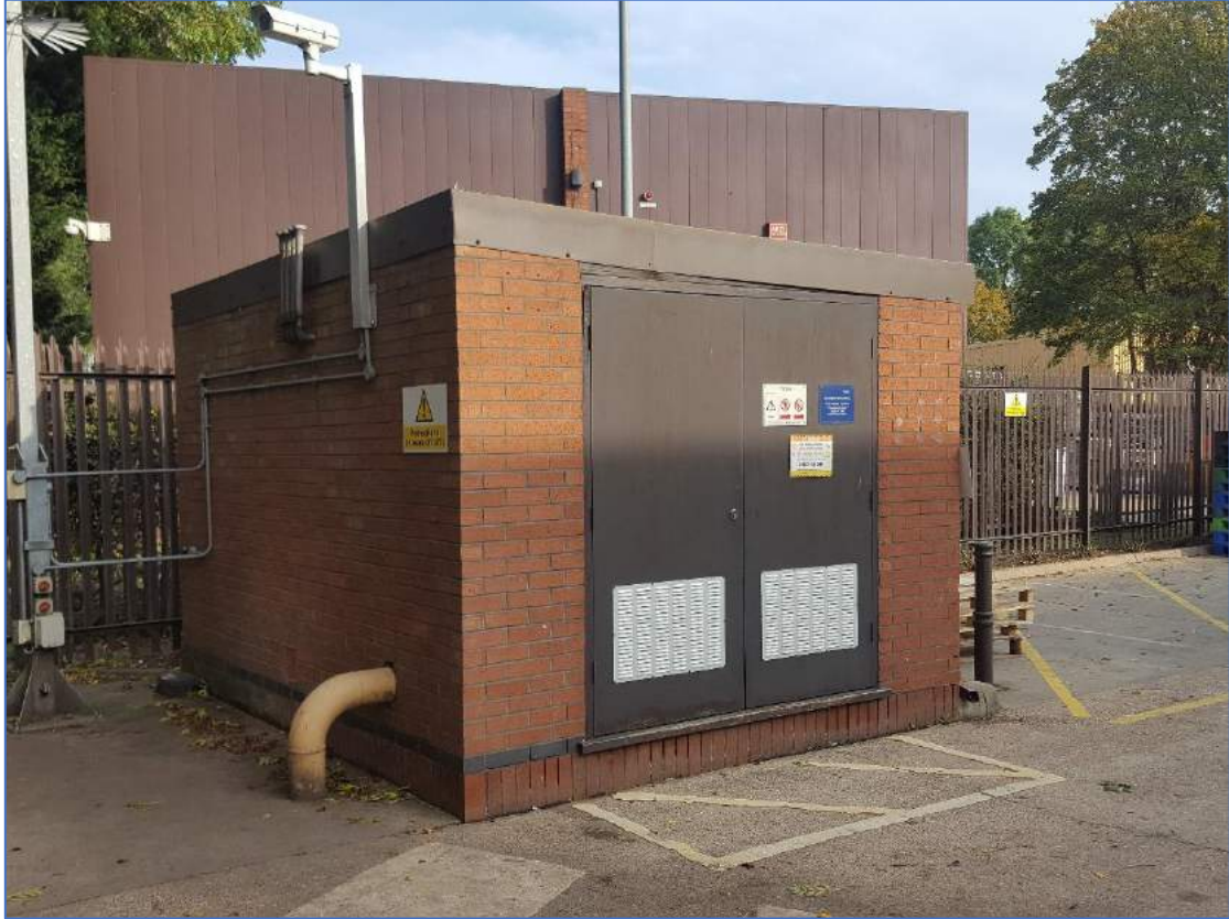
Photo 23 – Gas supply building
