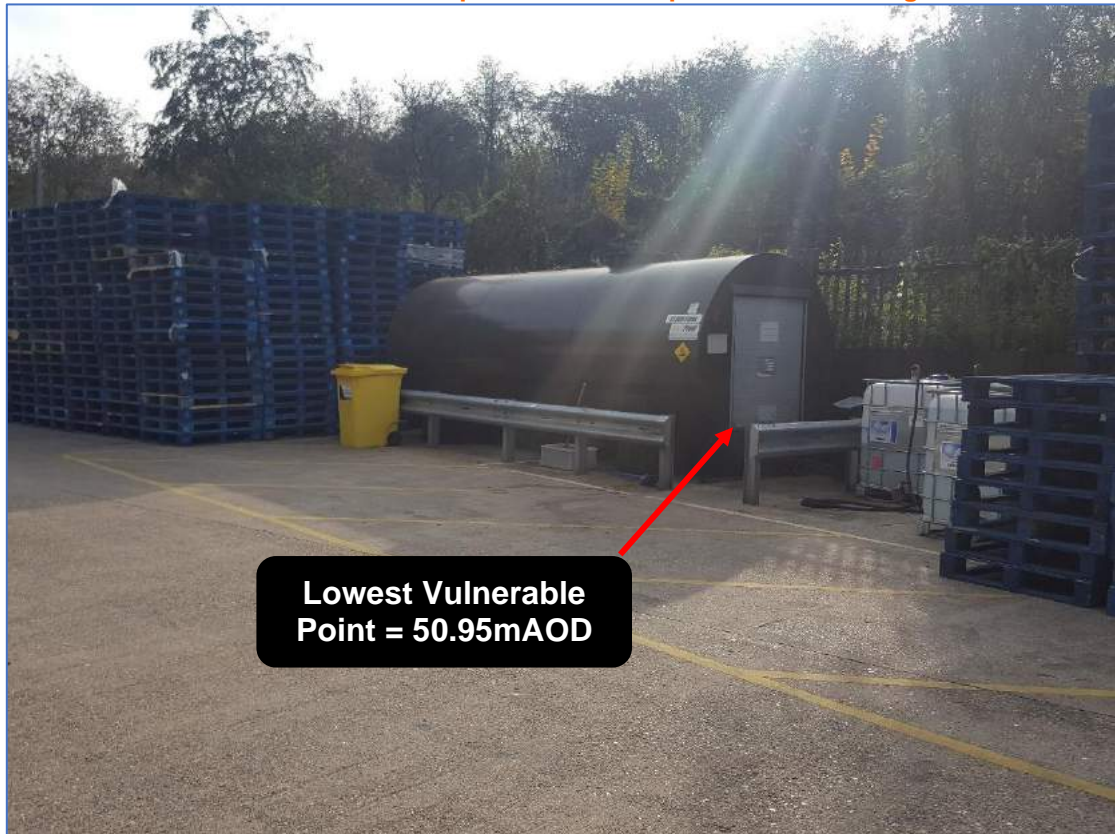
Photo 26 – Diesel tank on the southern perimeter of the production building
