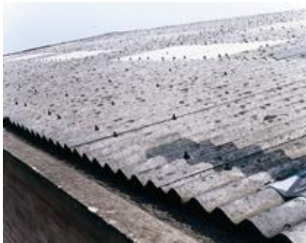
Asbestos Containing Roof
