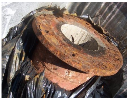
Scale within pipes/components (NORM)
