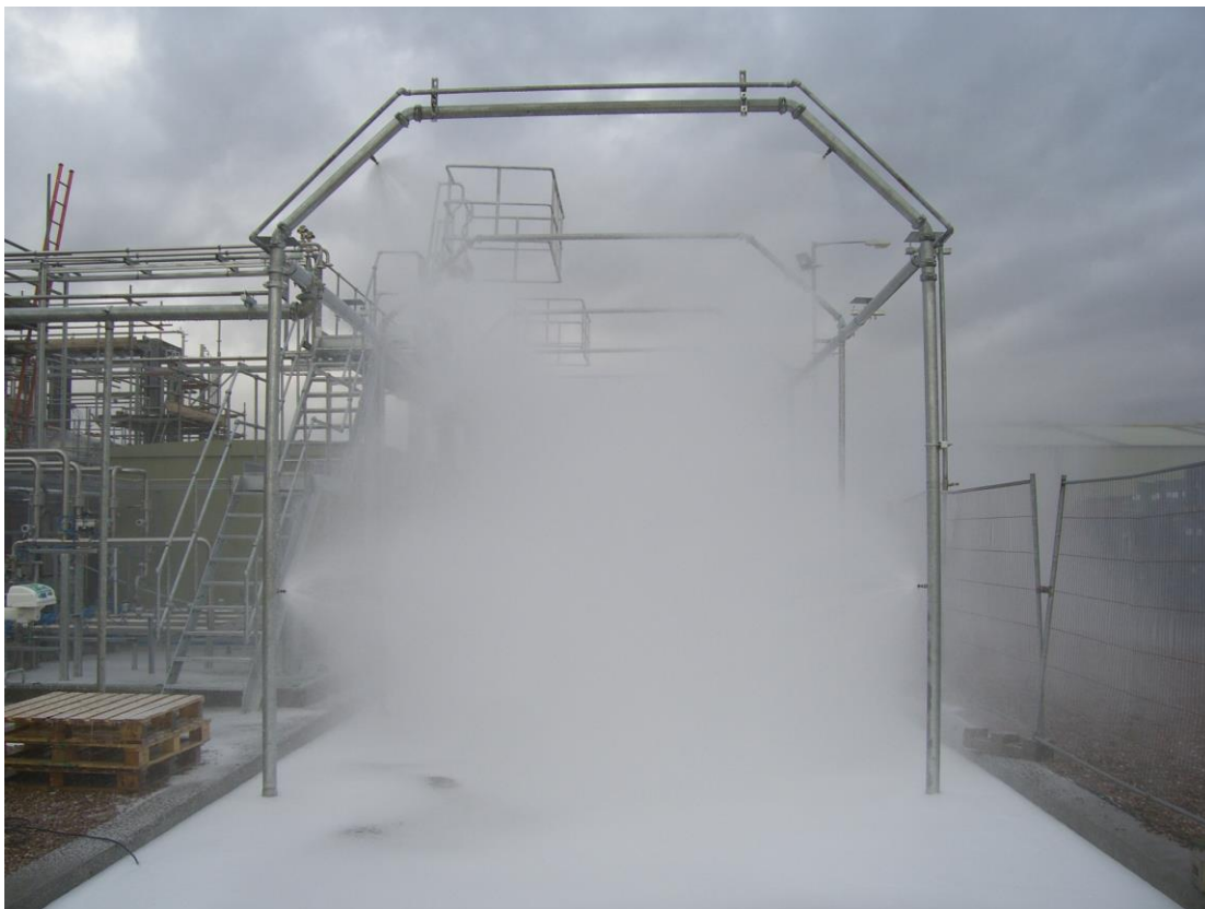
Typical tanker off-loading bay deluge/spray protection in operation
