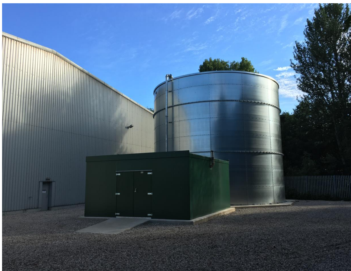
Typical water storage tank and GRP enclosure.
