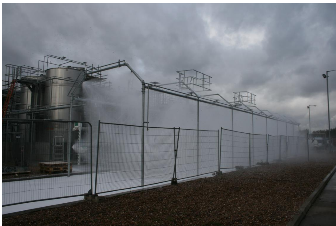
Typical tanker off-loading bay deluge/spray protection in operation
