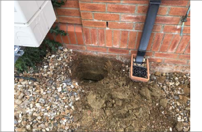
21: HDP4 left of drain
