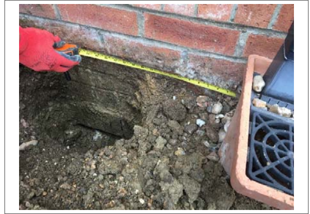
22: HDP4 left of drain
