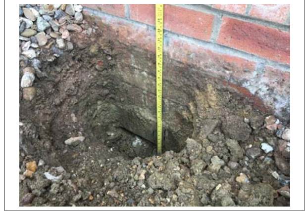
24: HDP4 left of drain
