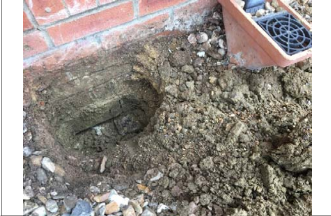
23: HDP4 left of drain
