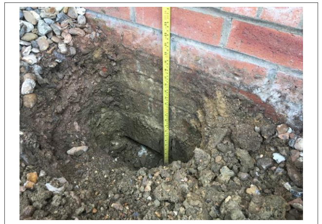
24: HDP4 left of drain
