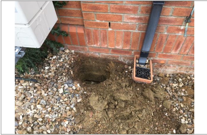
21: HDP4 left of drain
