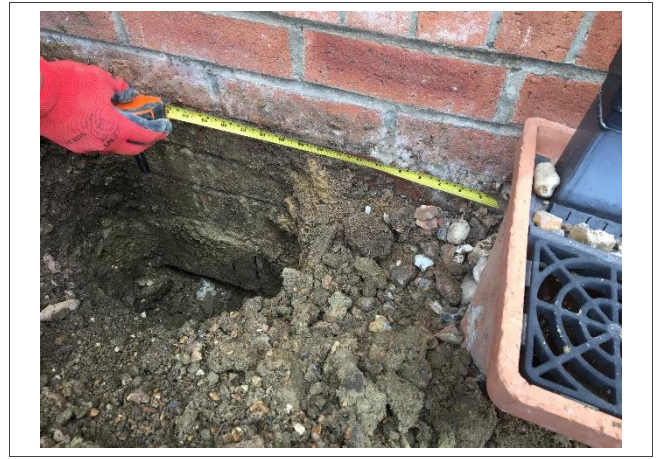
22: HDP4 left of drain
