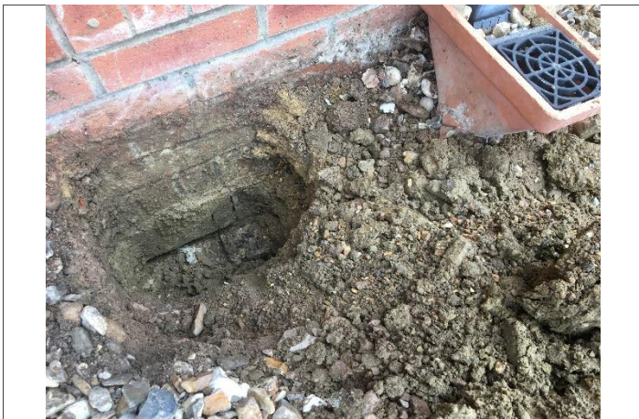
23: HDP4 left of drain
