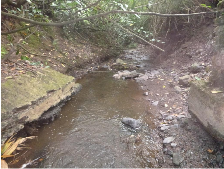
Figure 7: view looking downstream from underneath the footbridge (waterwheel to be cut into the bank on the left-hand side).
