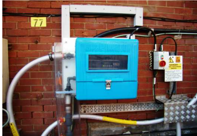
Figure J2 – Photograph showing the sodium hypochlorite dosing equipment - Hypochlorite is fed via double contained piping and valves to each of four dosing cubes incorporating the pump unit
