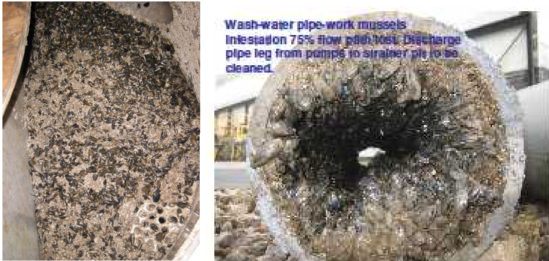
Only three out of circa 400 cooling tubes visible due to marine fouling.
