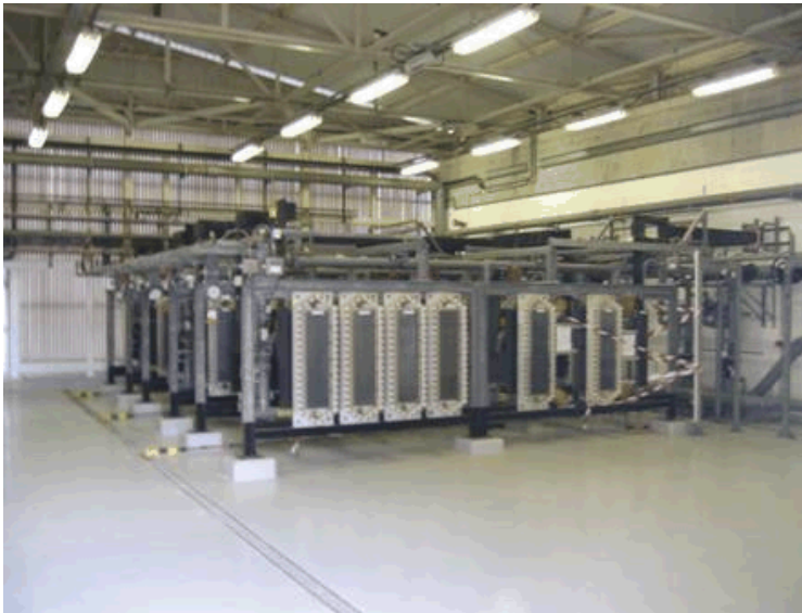
Figure J3 – Photograph of an electrochlorination plant
