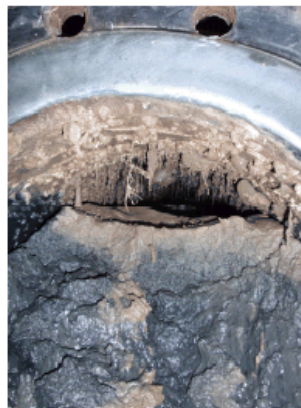
Figure C2 - A view of silt/sludge accumulation within pipework
