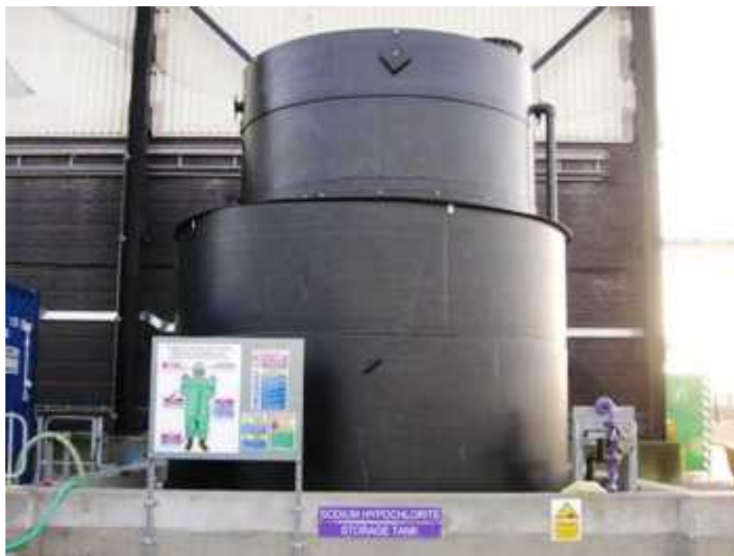
Figure J1 – Photograph of a sodium hypochlorite bulk storage tank at Heysham 2
