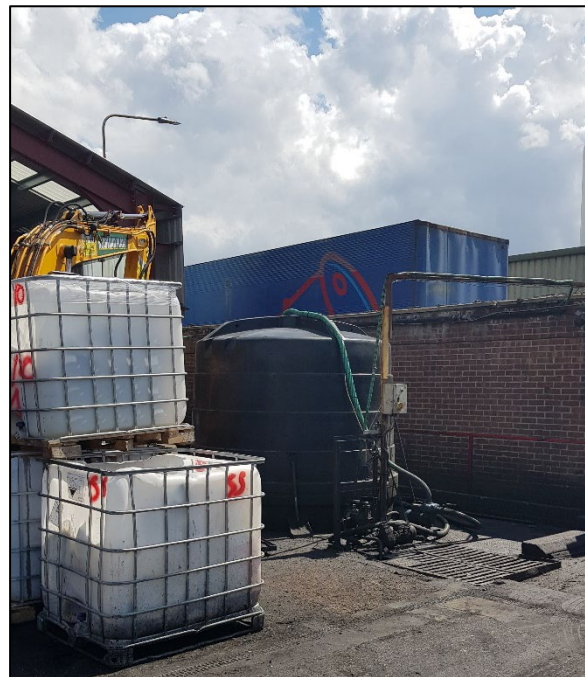
Figure ASR9: Rainwater Storage Tank in Bottom Yard
