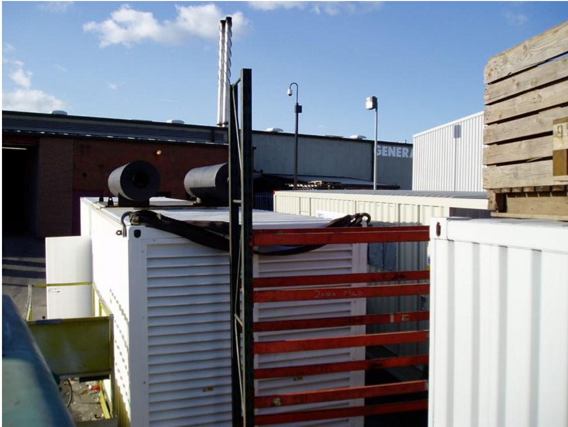
Figure 11.4: Example Generator Enclosure with High Specification Exhaust Silencers
