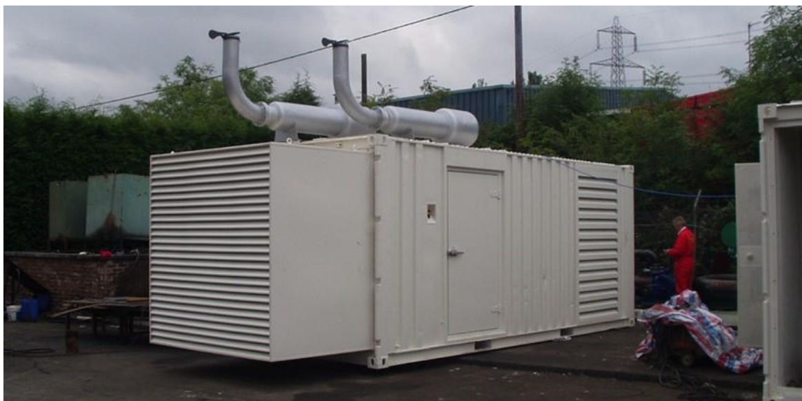
Figure 11.2: Mud Pump Engine Enclosure (note Exhaust Silencers)
