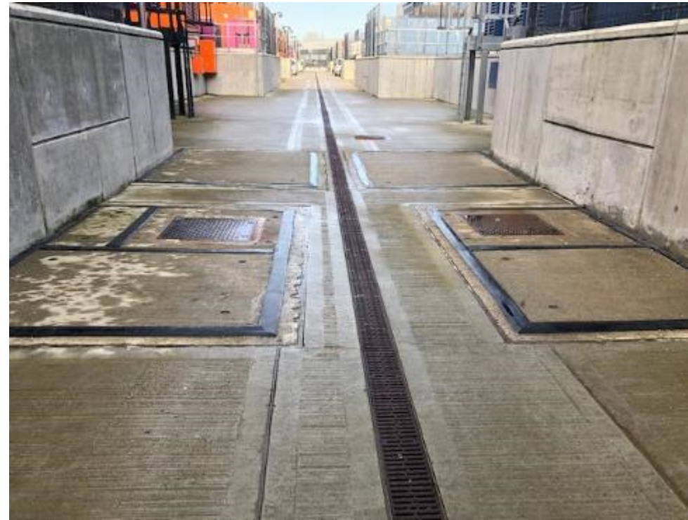
Photo 2: Campus - inside the permit area looking north. Note concrete AST bunds in the foreground of picture.
