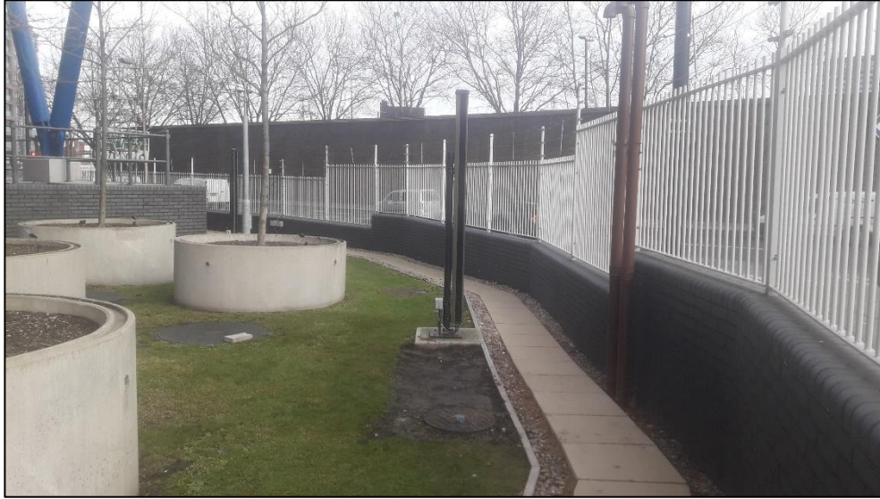
Photograph 1 – Area concerning the point of loss (07/01/2021)
