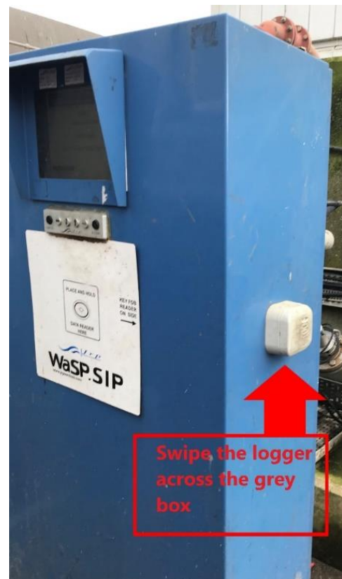
Figure 2: JRP Logger & swipe point
