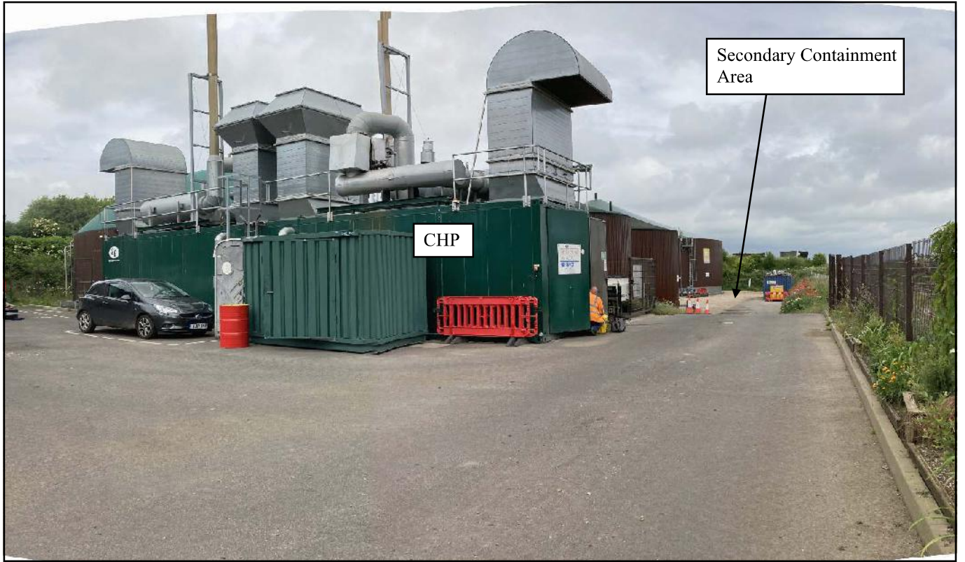
Photo 33. View of small hard standing area at a level above secondary containment area.
