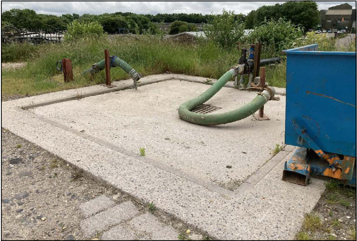
Photo 25. View of digestate draw-off point and spill collection drain.
