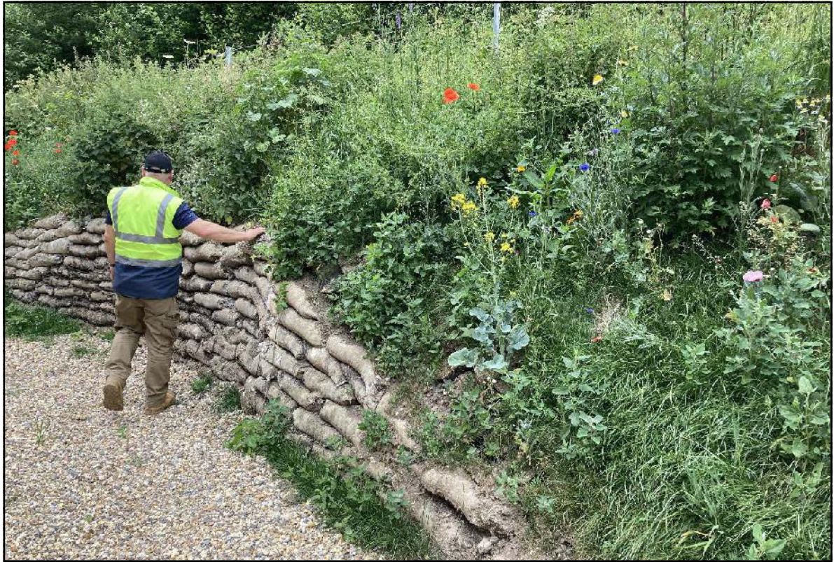
Photo 29. View of northern margin showing detail of concrete sandbag wall retaining GCL.
