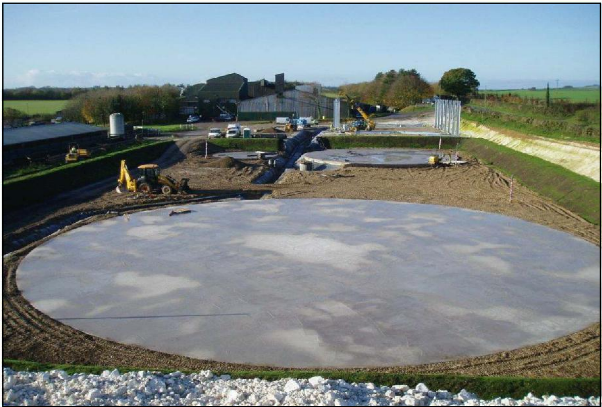
Photo 14. View looking west of concrete tank bases, grassed sideslopes, pipe work trench / Sump and aggregate covered GCL.
