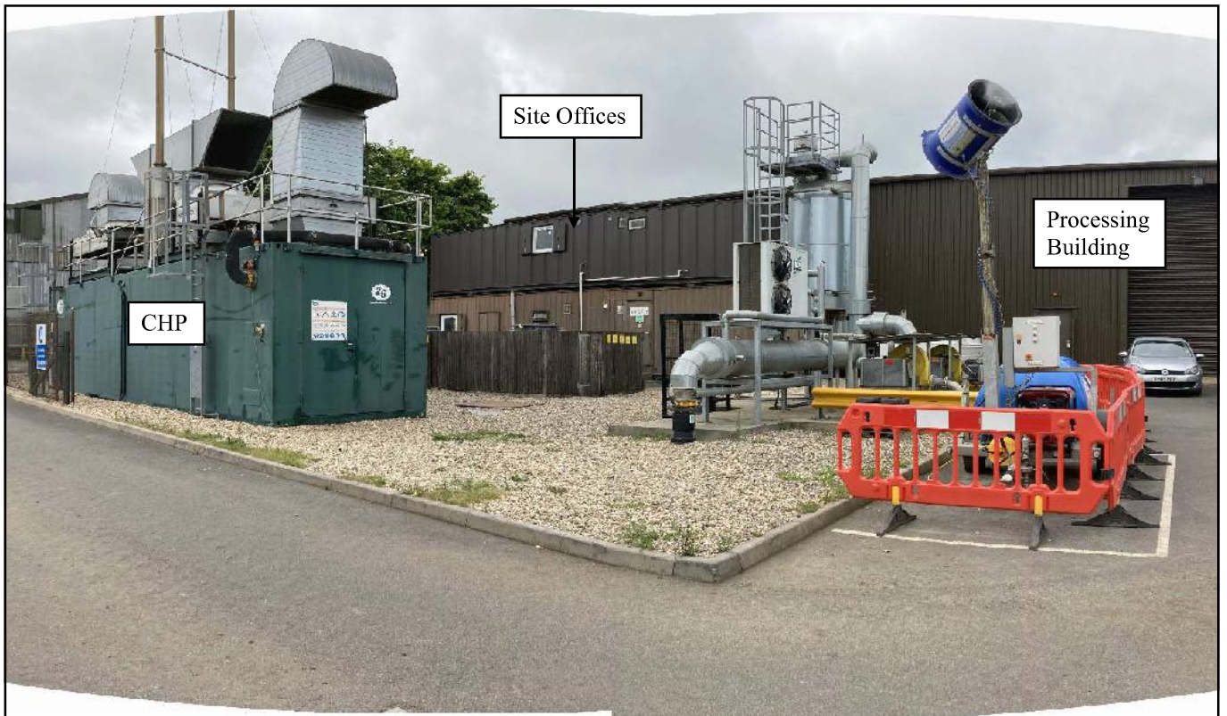
Photo 32. View of small hard standing area at a level above secondary containment area.
