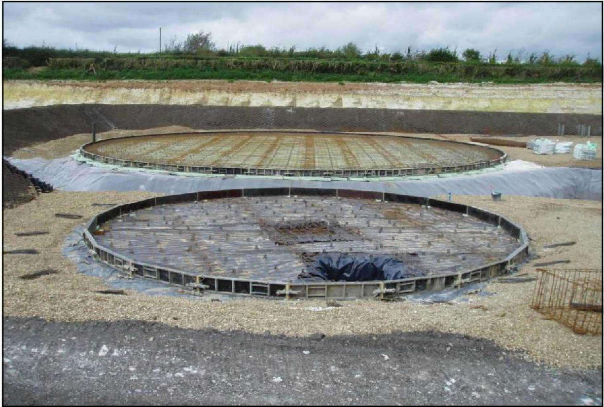
Photo 7. Reinforced concrete tank bases being laid over the top of the GCL.
