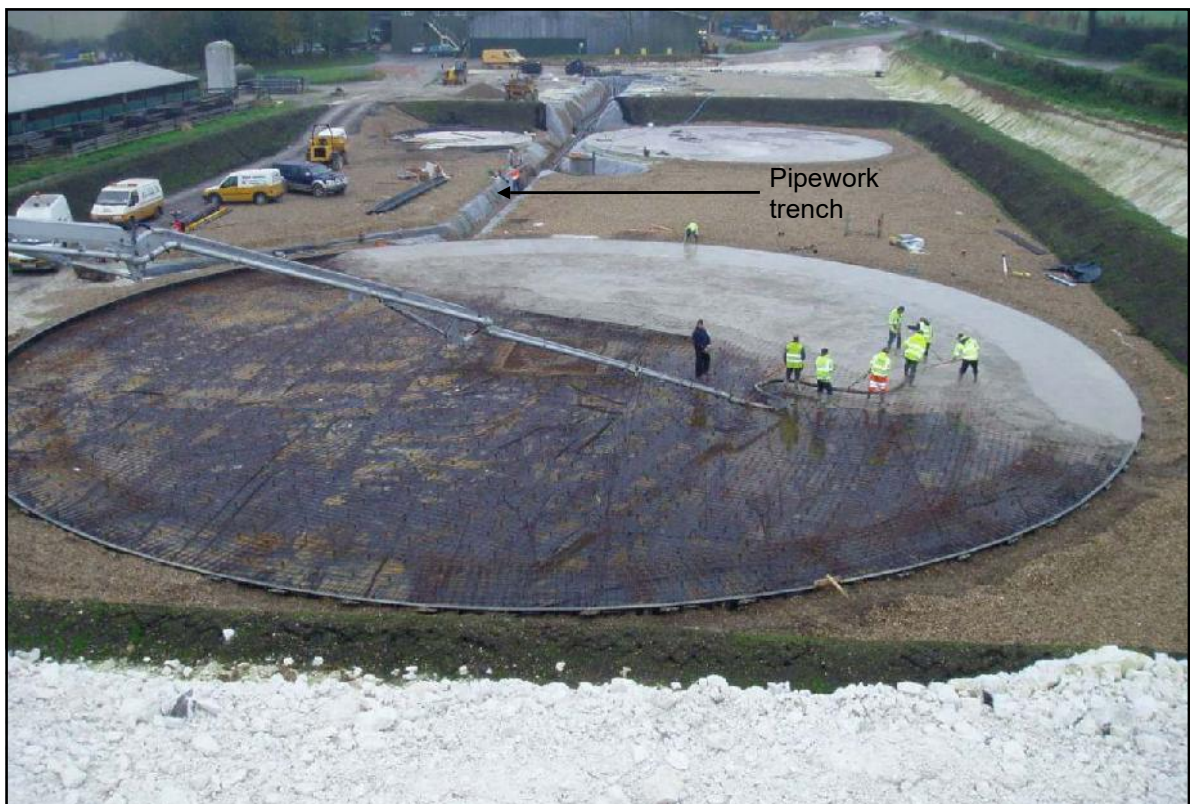
Photo 10. Reinforced concrete tank base for Digestive Storage Tank being laid and pipe work being installed.
