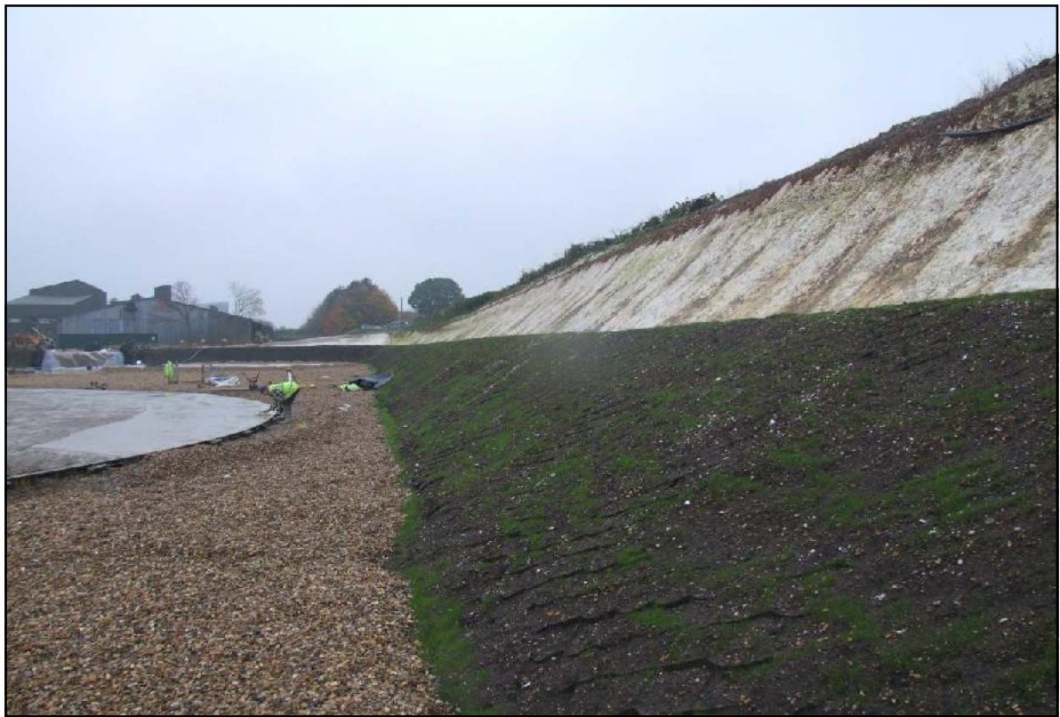
Photo 6. GCL secured on sidewall with “Envirogrid” filled with soils. View of northern slopes.
