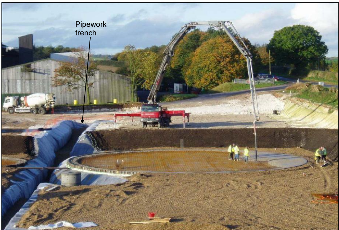
Photo 8. Reinforced concrete tank bases being laid over the top of the GCL.
