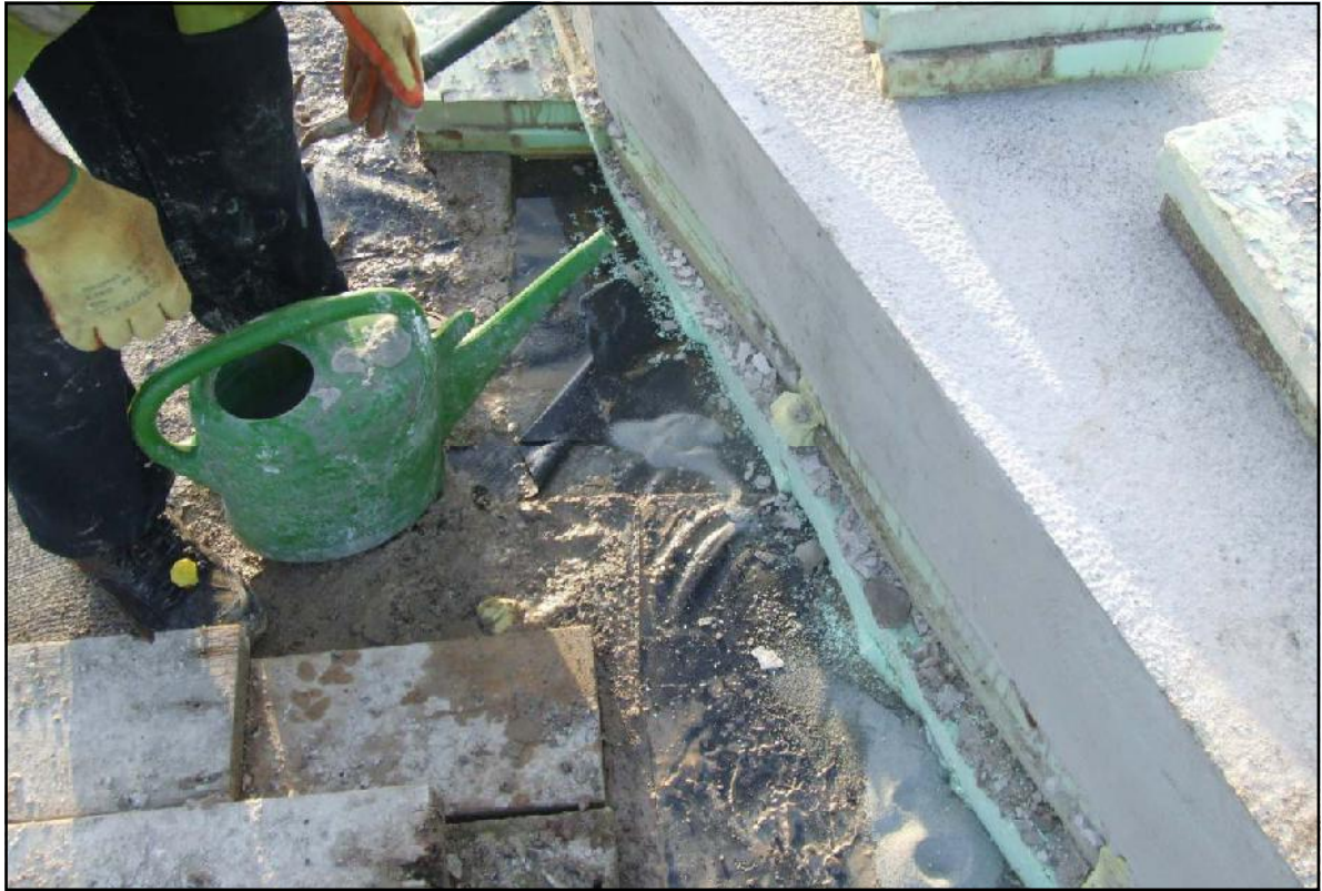
Photo 9. Holes in GCL from concrete shutter pins sealed with bentonite powder.
