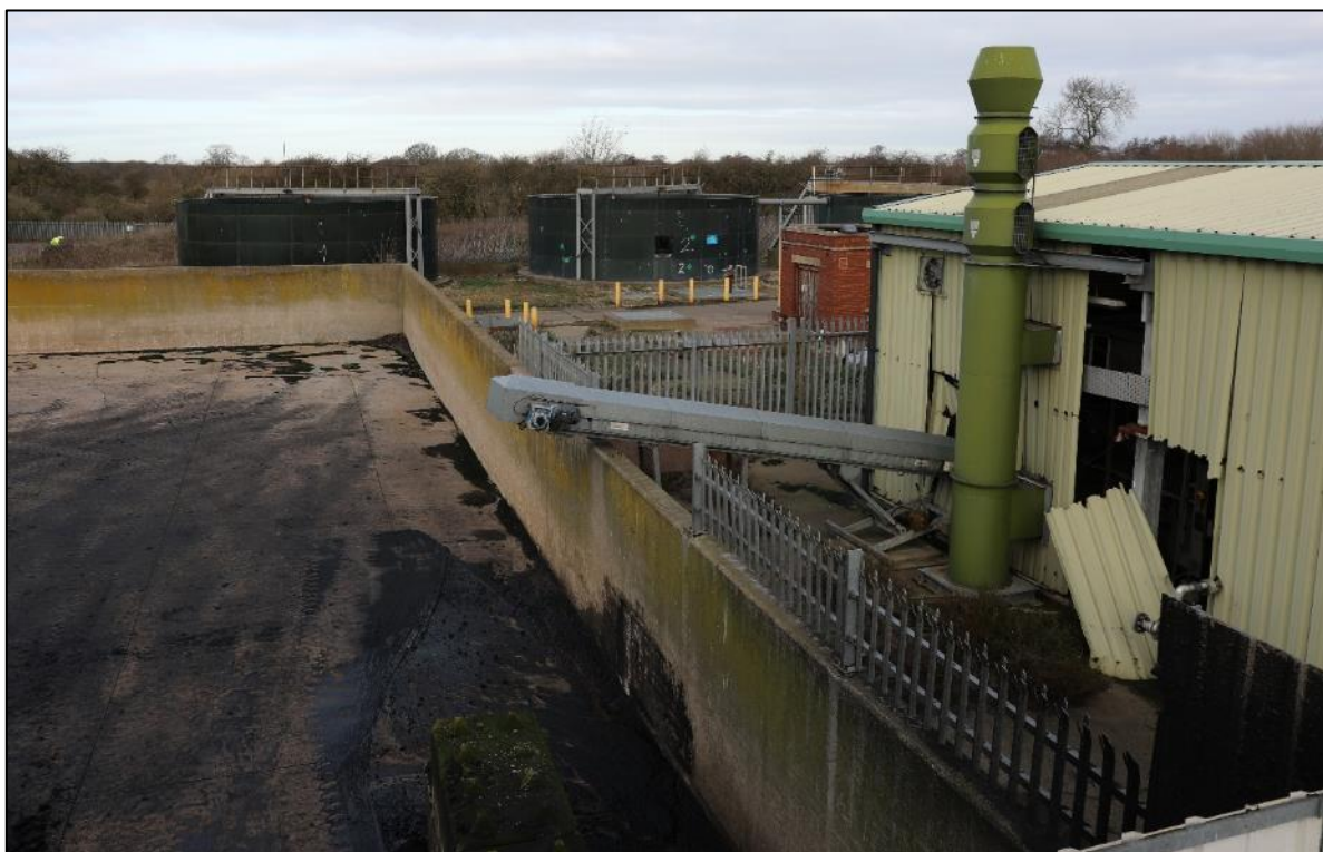
Figure 17. Sludge cake conveyor and pad.
