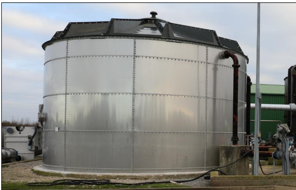
Figure 10. Imported sludge buffer tank.
