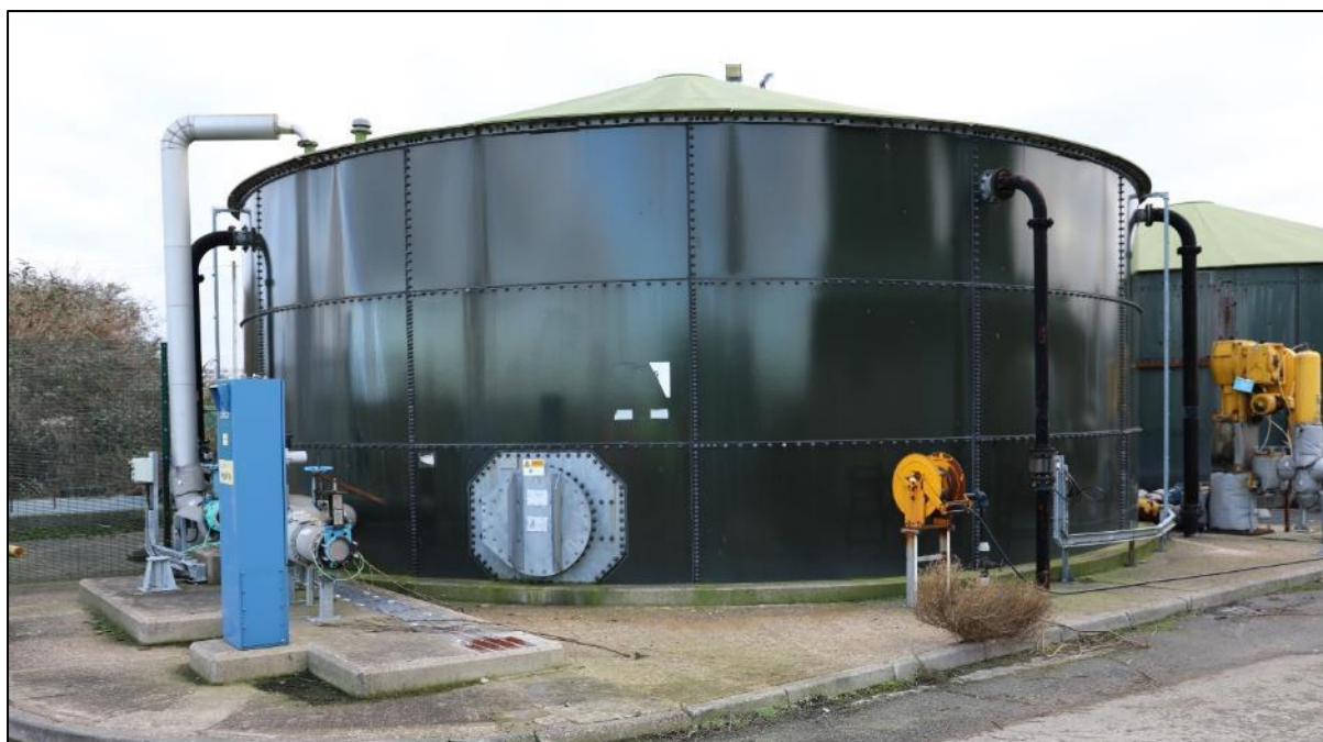
Figure 13. Sludge blending (digester feed) tank.
