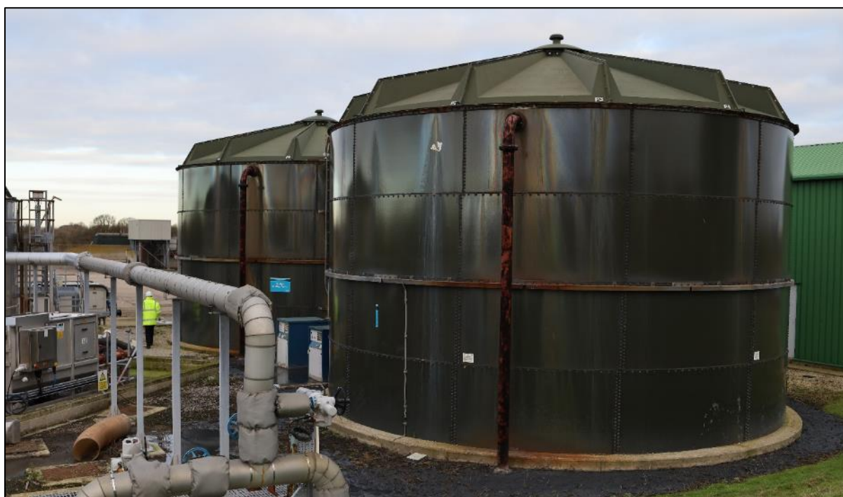
Figure 11. Imported sludge holding tanks (2 no.).
