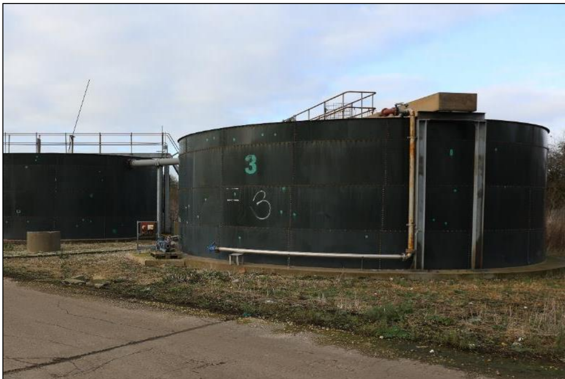
Figure 15. Dewatering feed tank (on the right).
