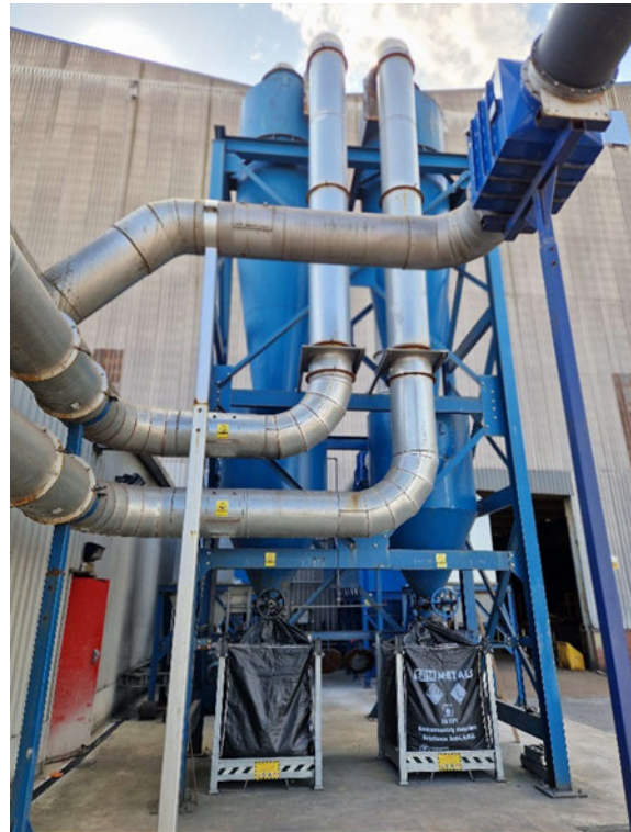
Figure 8: Cyclone filters for spray booth 1 (left) and 2 (right)
