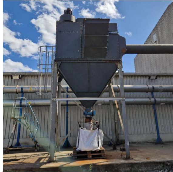
Figure 6: Dust collector for grit blaster
