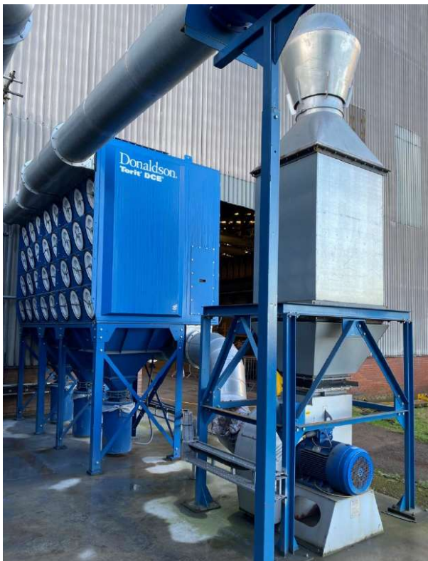
Figure 7: Spray booth 1 dust collector and emission stack A134a
