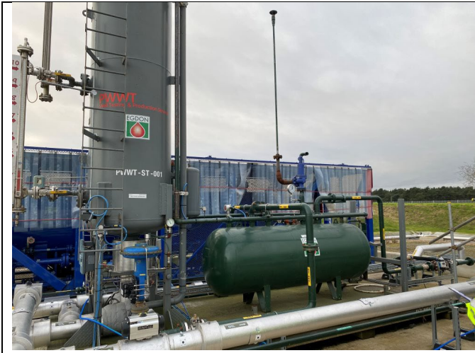
Piping connected to 2 nd stage separator on wellsite
