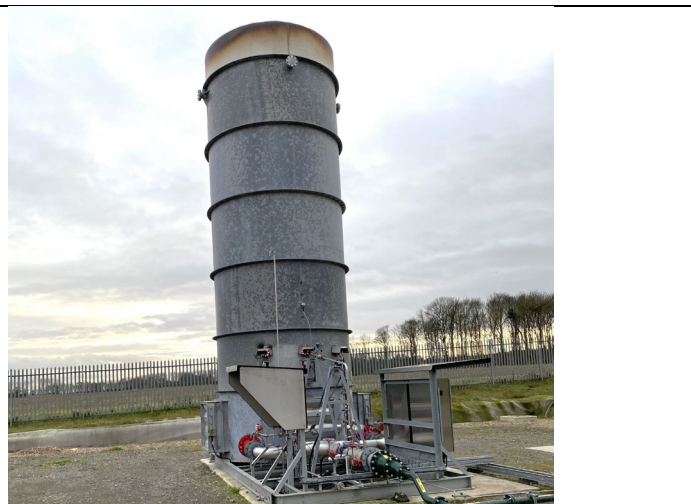
Enclosed ground flare on wellsite
