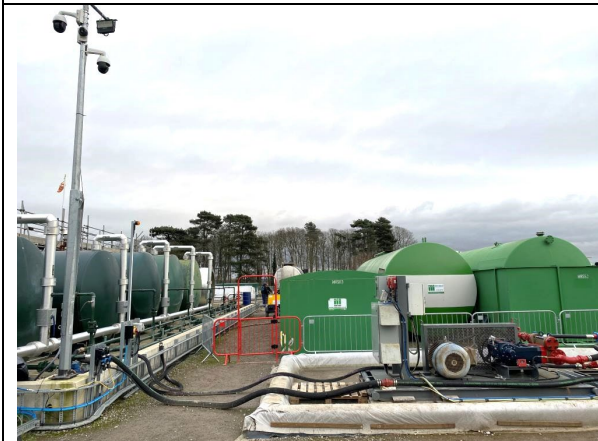
Liquid storage tanks on wellsite
