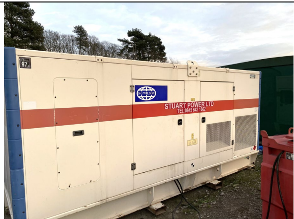
Acoustically enclosed packaged generator labelled LwA 97dB on wellsite
