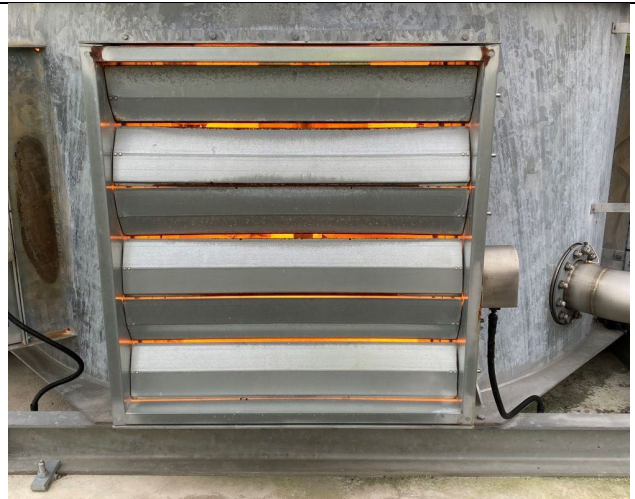
Close to an inlet aperture (90% closed) of Enclosed Ground Flare on wellsite
