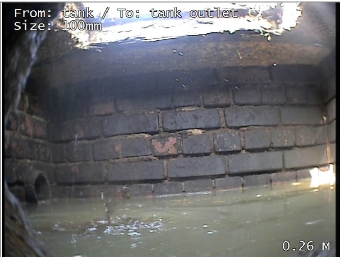
Finish node type, manhole, reference tank outlet
