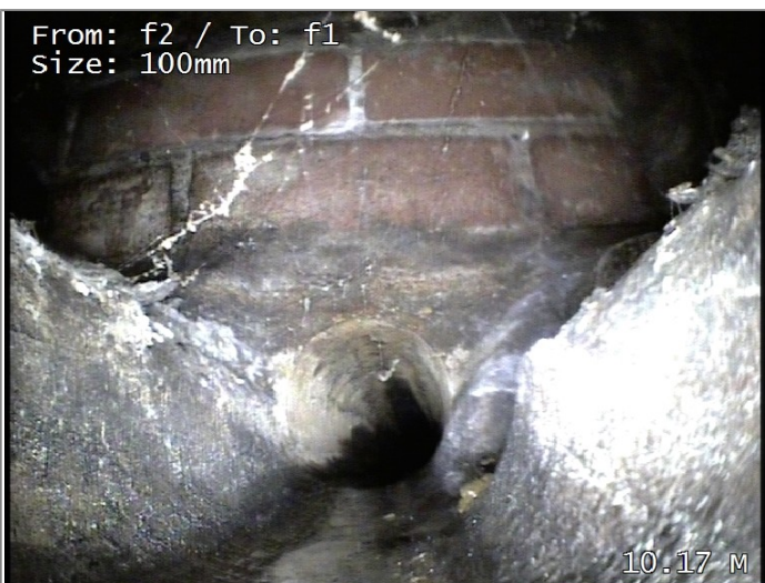
Finish node type, manhole, reference f1
