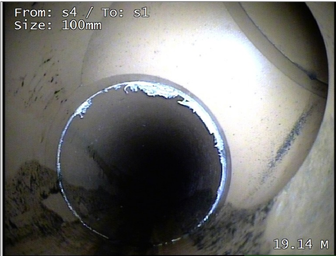
Connection other than junction at 1 o'clock, diameter 100mm
