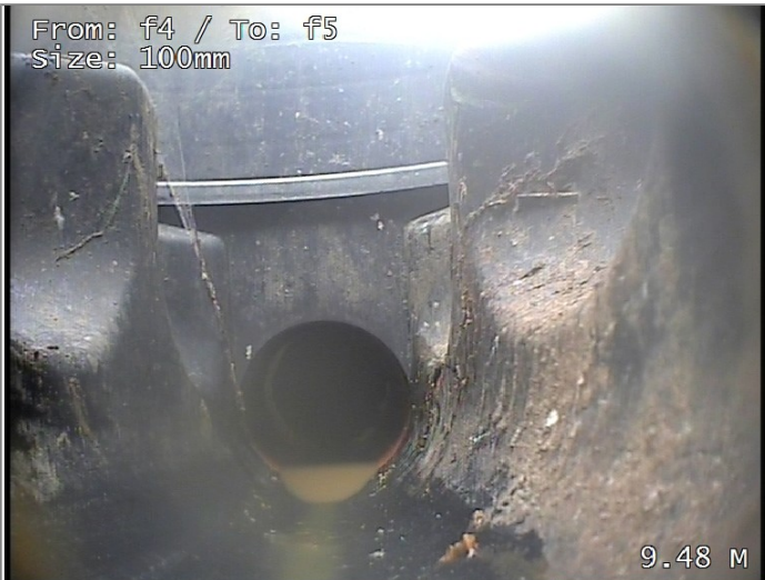
Finish node type, manhole, reference f5
