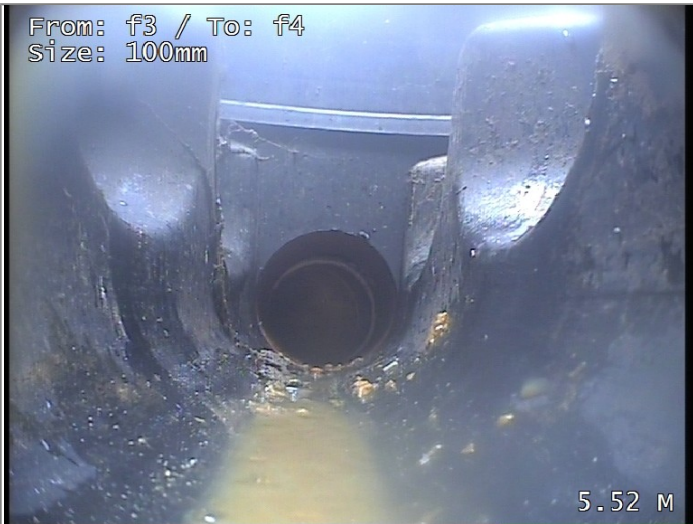
Finish node type, manhole, reference f4
