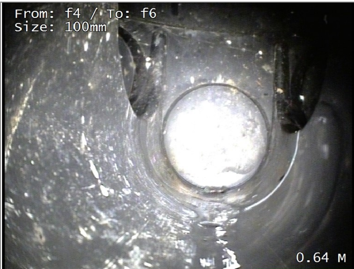
Finish node type, manhole, reference f6
