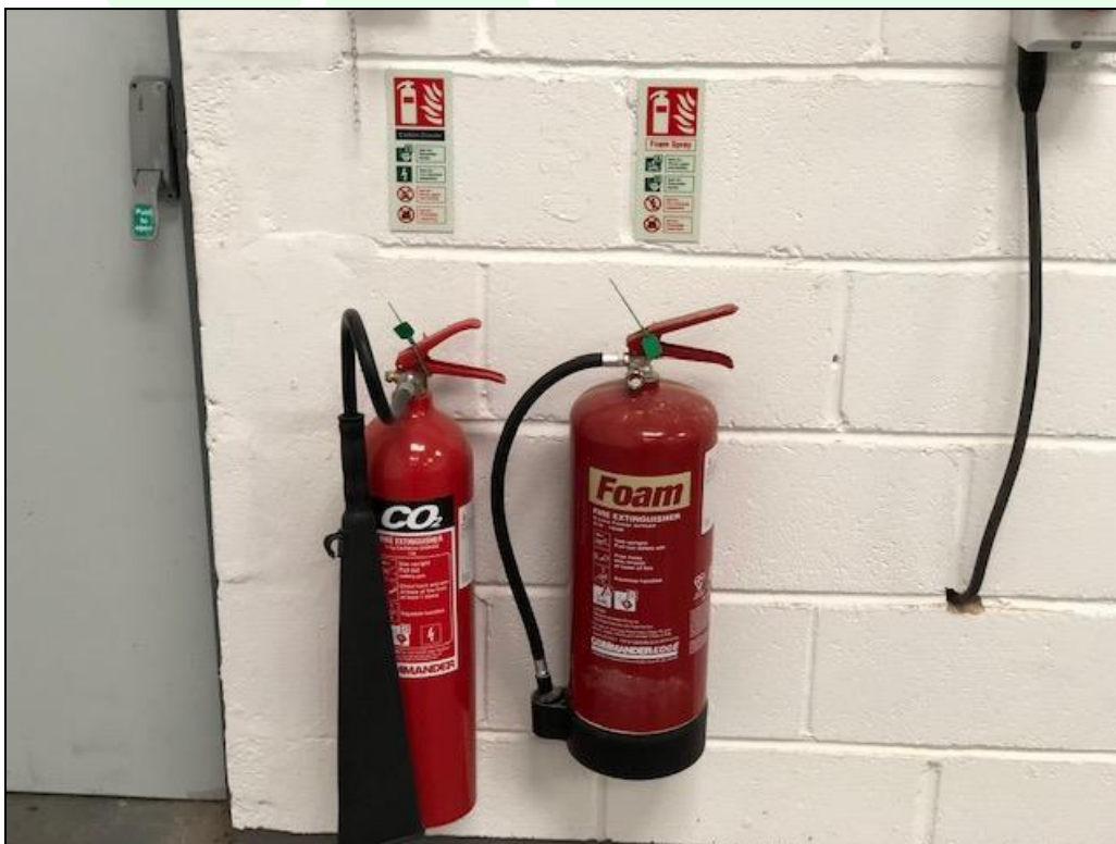
Figure 5 Manual Fire Extinguishers
