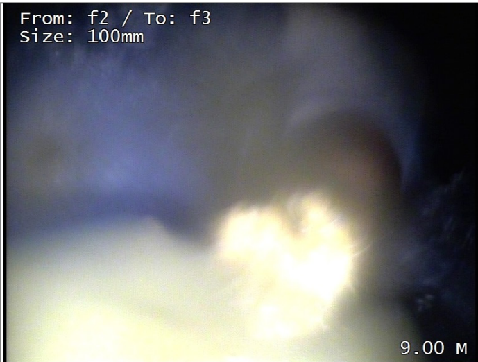
Finish node type, manhole, reference f3
