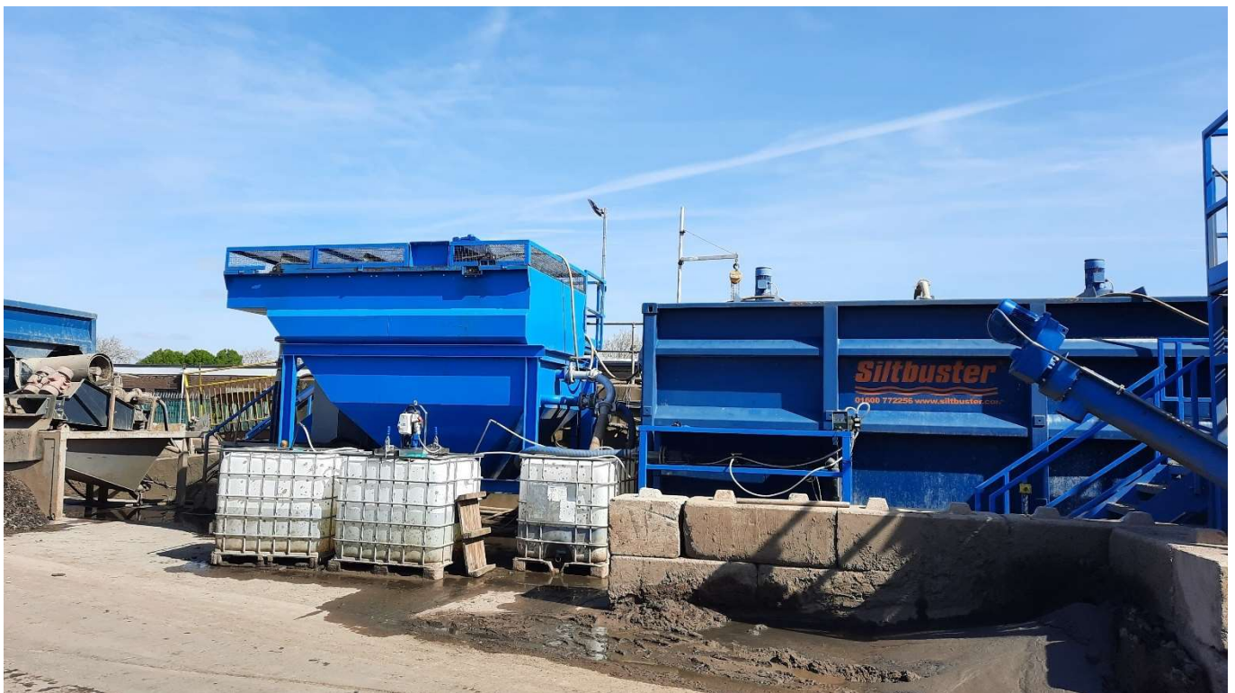
Figure C.4: New Wet Waste Dewatering Plant
