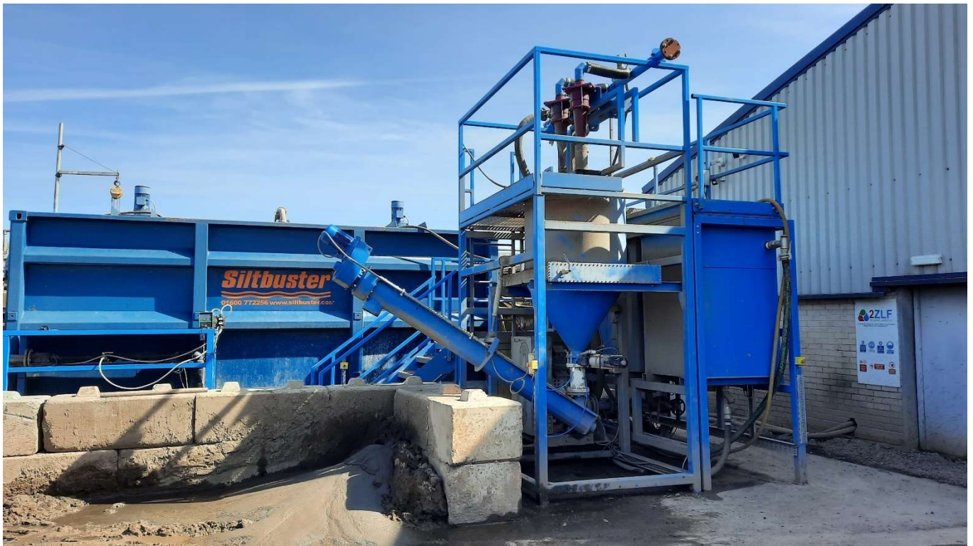
Figure C.3: New Wet Waste Dewatering Plant
