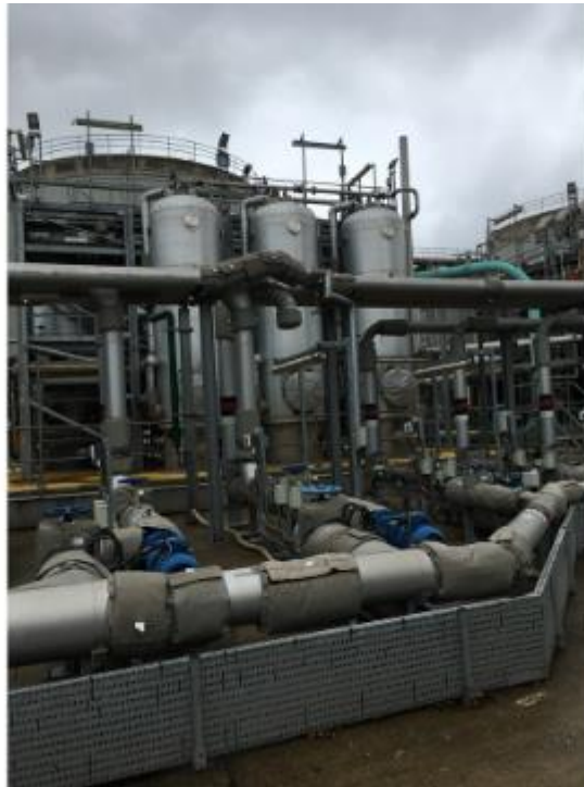
Photo of one of part of the THP process. Pre-treated sludge is transferred to the primary digester tanks.
