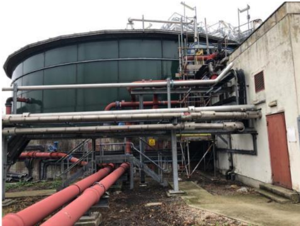
Photo of the main dewatering press buffer tank. Digested sludge is transferred for dewatering within the cake barn.
