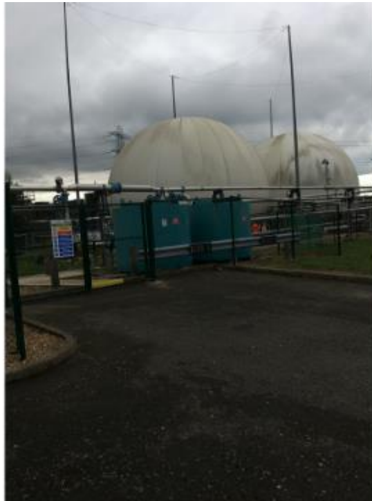
Photo of the two gas holders. Siloxane filters can also be seen on the biogas line.
