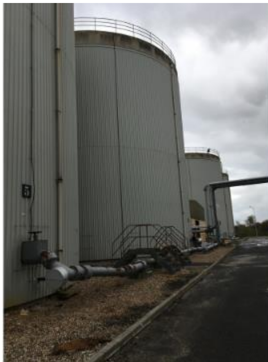
Photo of primary digester tanks on site. Digested sludge is transferred to the secondary digester tank. Biogas is transferred to the gas holders.
