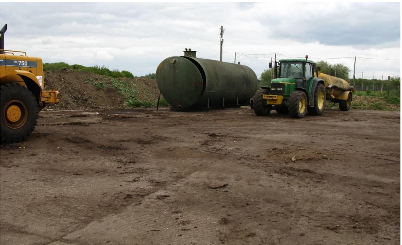
The photograph above shows the concrete pad at the location for the proposed development, together with the start of the construction of the screening bund to the north. This is newly placed soil. Most of the redundant plant have been removed from site.
