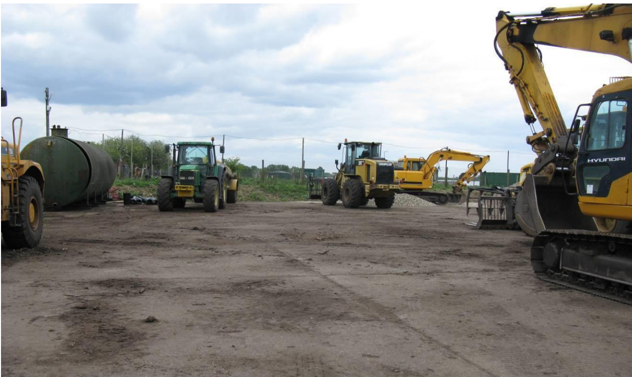
Photograph looking north-east across the concrete pad at the proposed development location dated 6 th May 2019.
