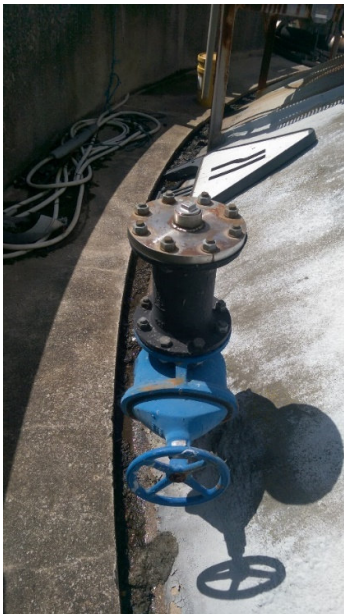
Chemical dosing point
