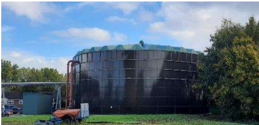
Photo 10: Post Digestion tank
