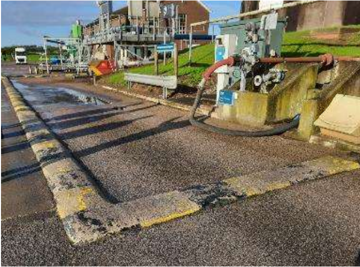
Photo 3: Raw sludge import point
