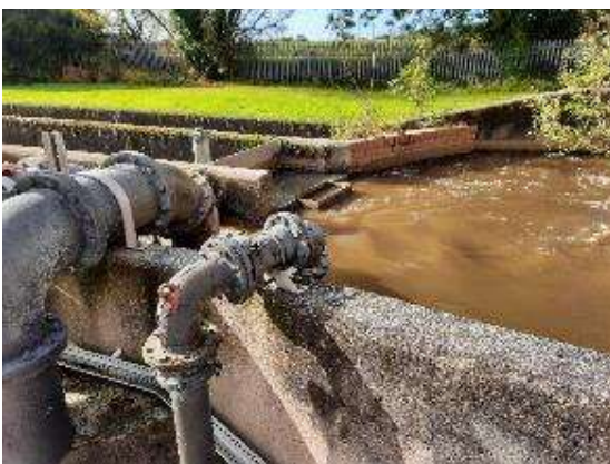
Photo 15: Centrate discharge point to head of works
