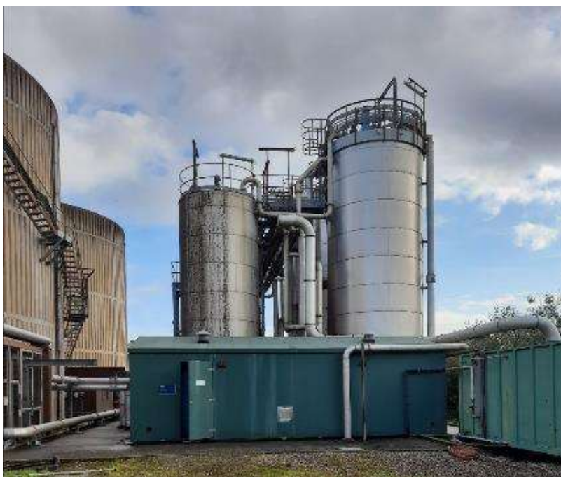
Photo 8: Thermophilic Aerobic Digesters
