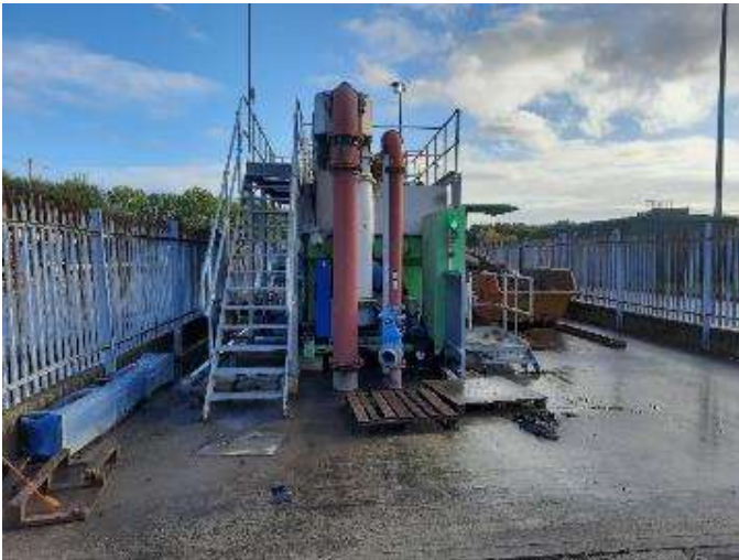
Photo 4: Sludge screening unit
