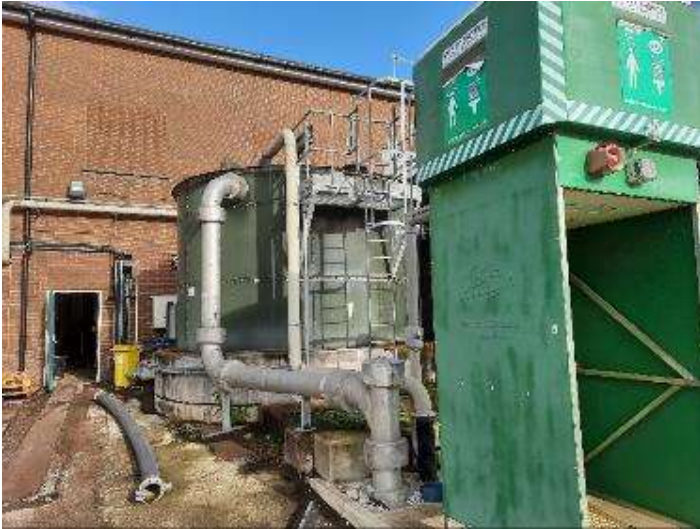
Photo 11: Digested sludge buffer tank
