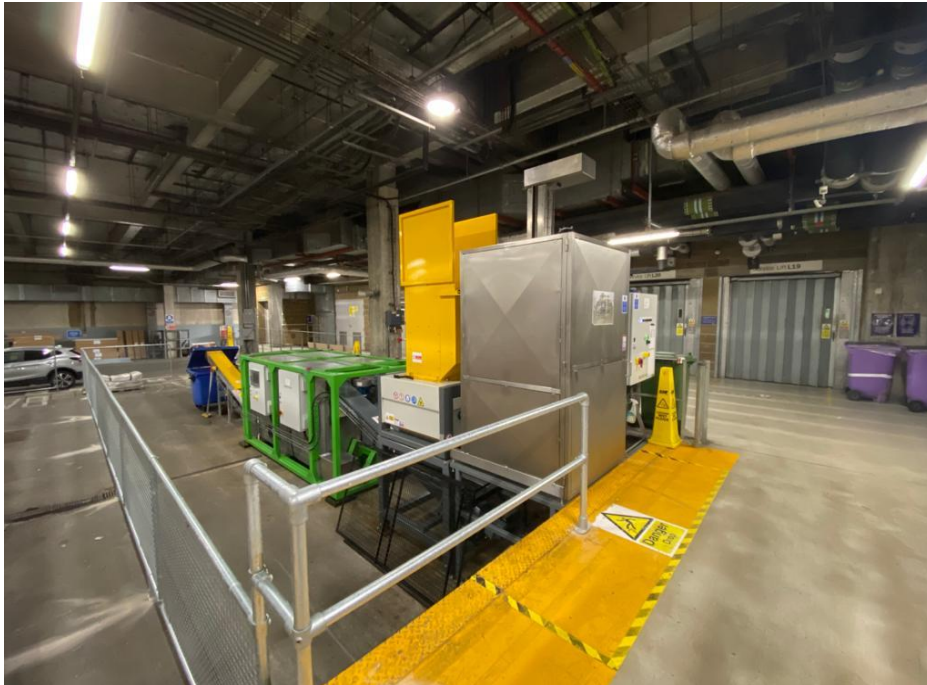
Figure 3 - Advetec Installation at Cribbs Causeway
