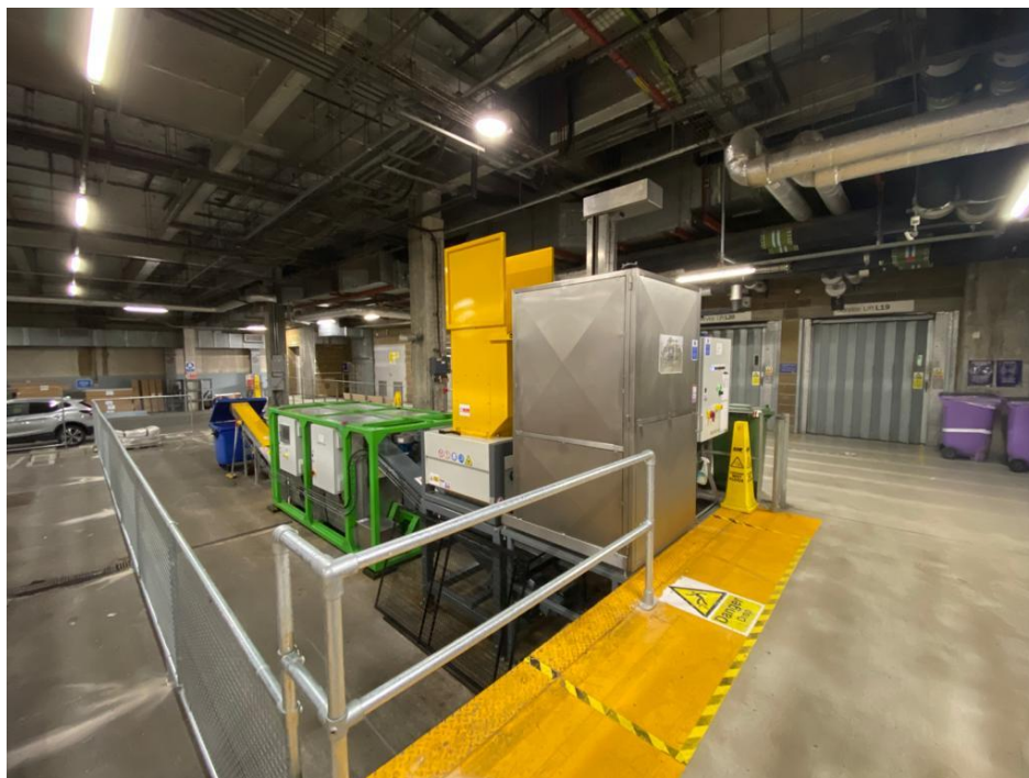
Figure 3 - Advetec Installation at Cribbs Causeway
