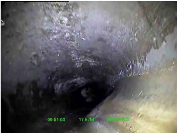
FJ00277624_STORM ENERGIA WORLE QUARRY_WORLE_5_005.jpg, 00:01:44, 17.57 m Deformed sewer or drain, 10%
