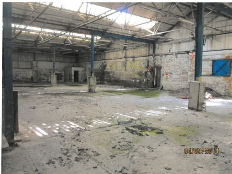
Picture 9: Inside vegetation treatment building.
