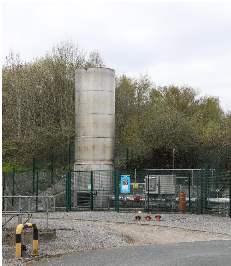
Figure J Waste gas burner
