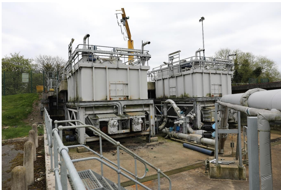
Figure E Sludge cake reception facility
