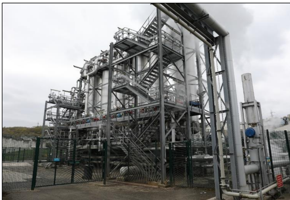
Figure 14. Thermal hydrolysis plant (THP).
