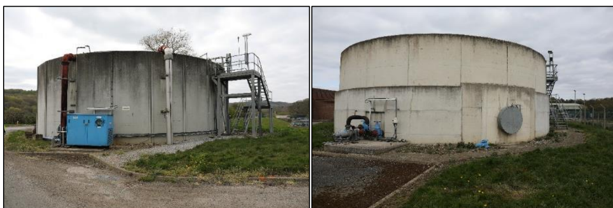
Figure 20. Conditioning feed tanks.
