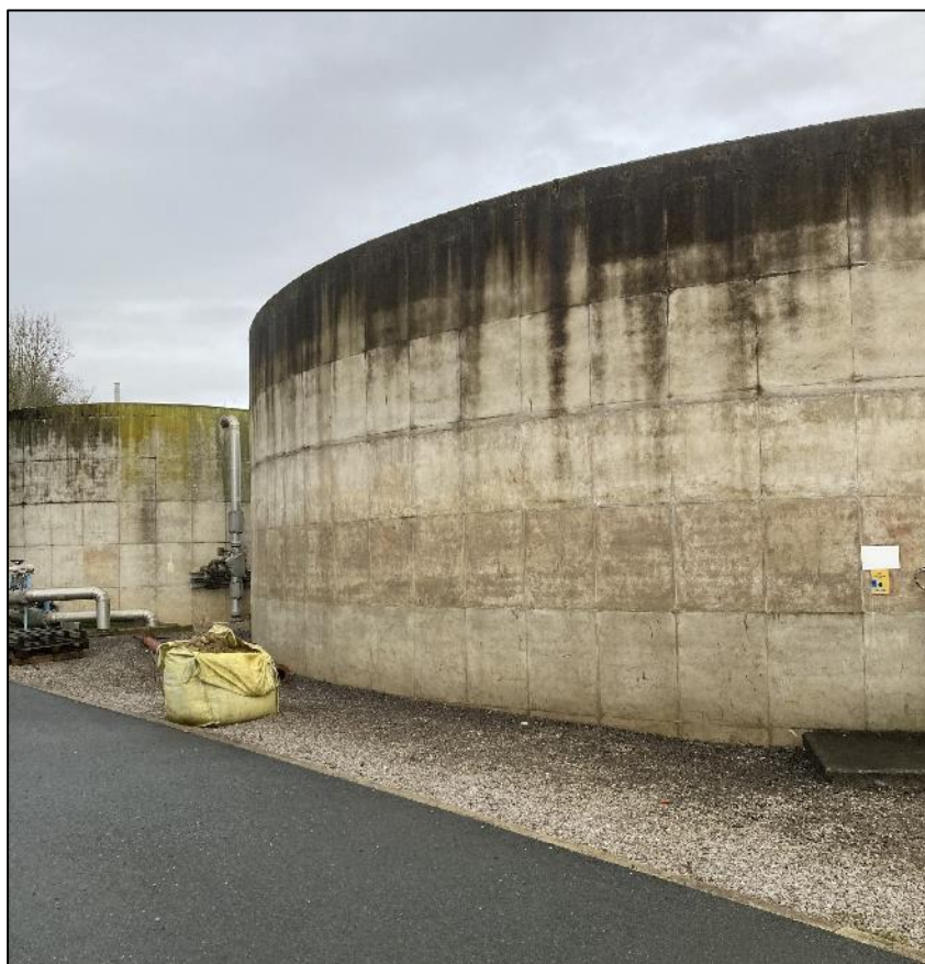
Figure 11. SAS storage tanks.
