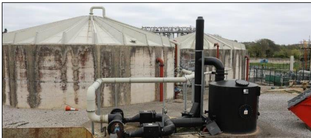
Figure 13. Mixed sludge tanks.
