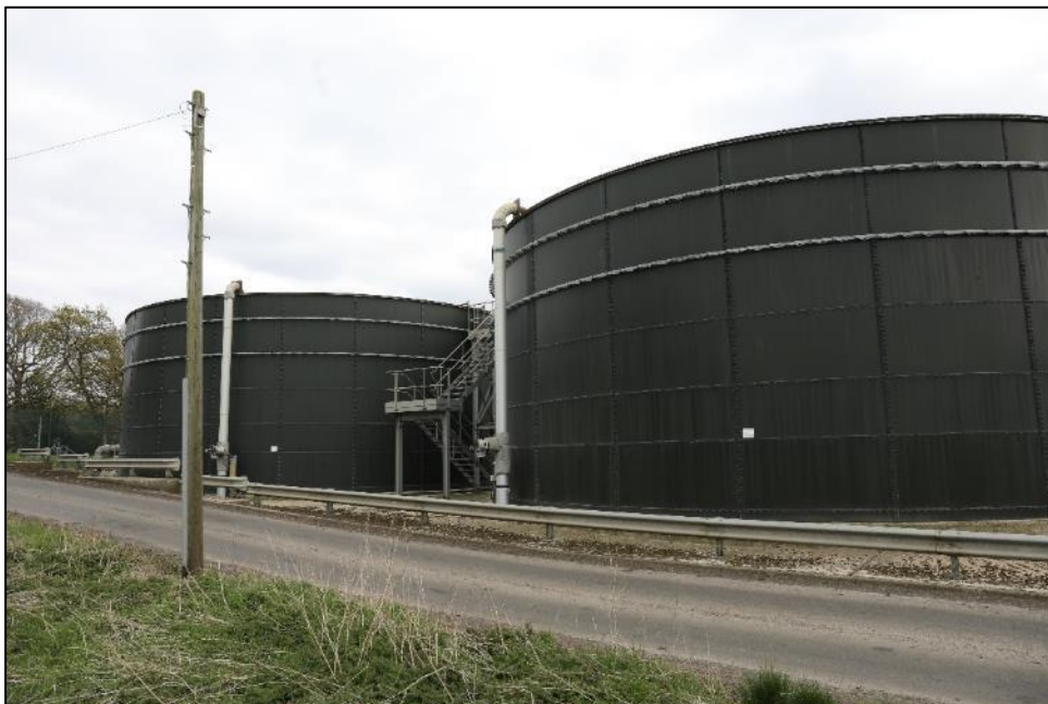
Figure 18. Export dewatering feed tanks.
