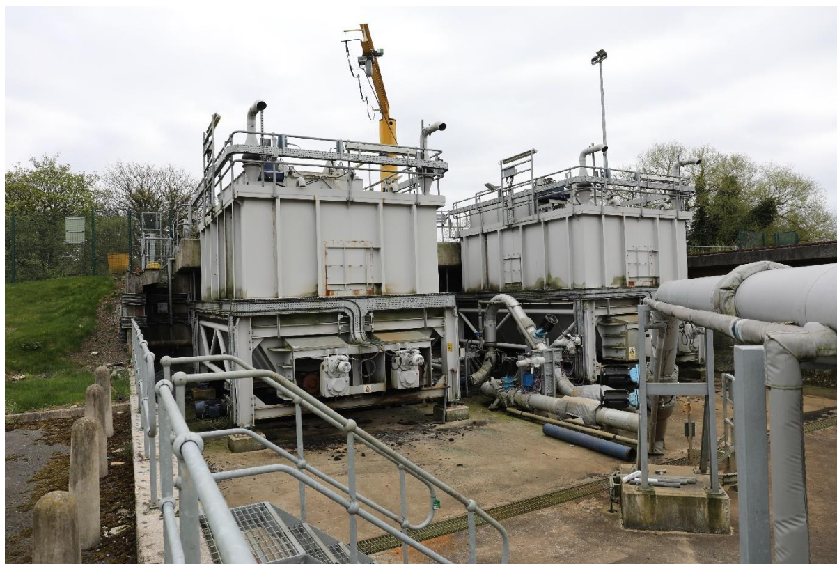
Figure E Sludge cake reception facility
