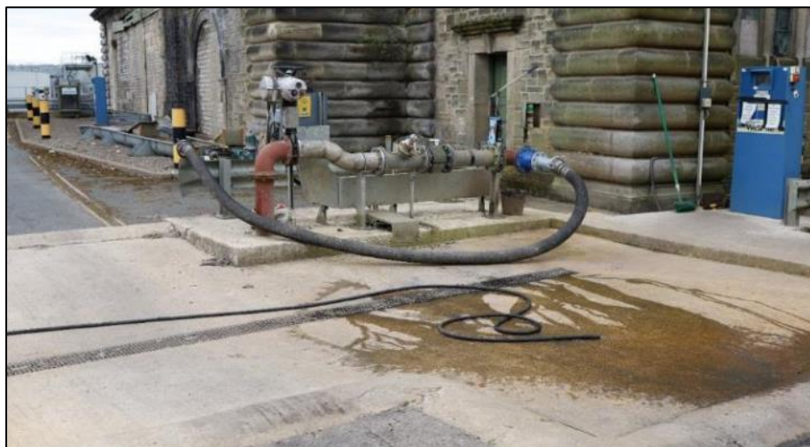
Figure 8. Sludge unloading area via WaSP loggers.
