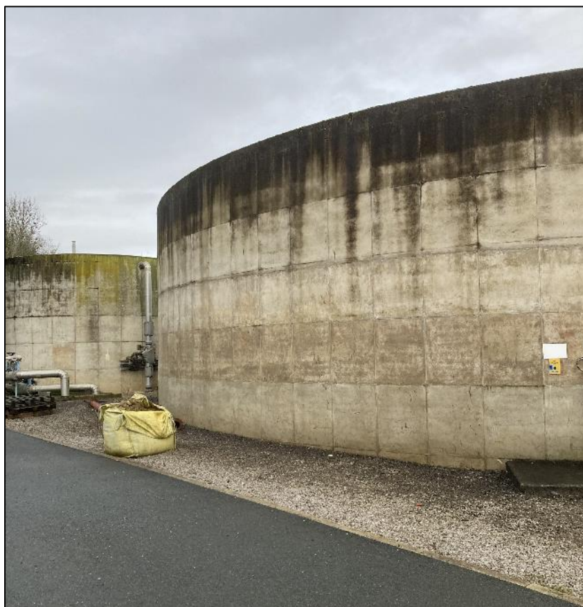
Figure 11. SAS storage tanks.
