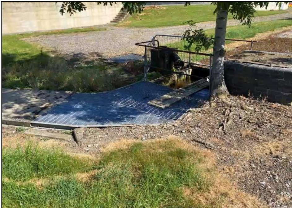
Figure 35. Sections of open decking on the channel feeding the humus tanks in the DW area (west).
