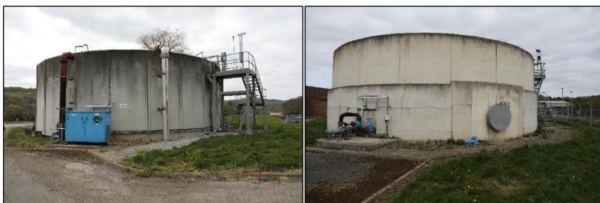
Figure 20. Conditioning feed tanks.
