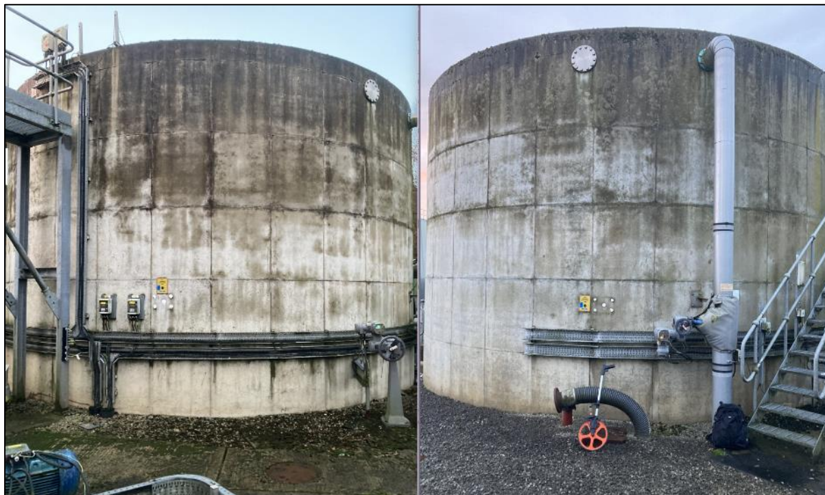
Figure 12. SAS transfer tanks (side by side images).
