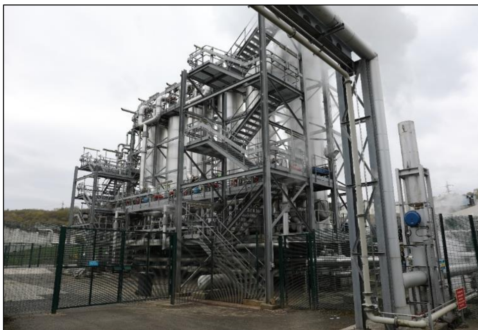
Figure 14. Thermal hydrolysis plant (THP).
