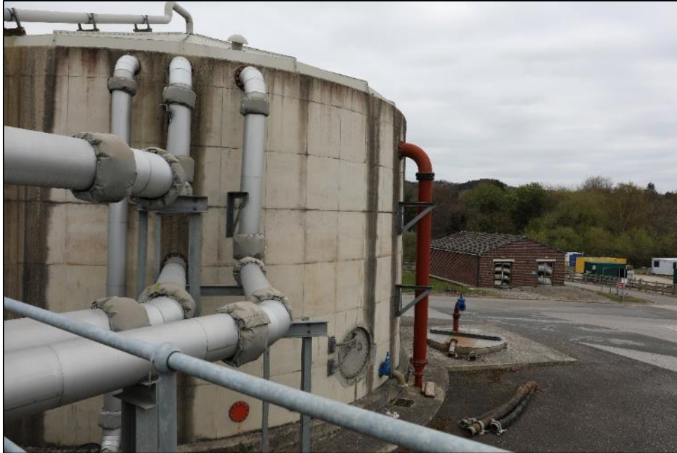
Figure 9. Sludge screen feed tank.
