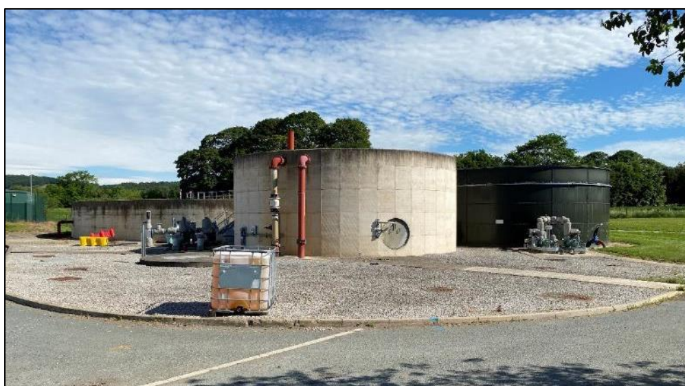
Figure 21. Centrate balance tanks.
