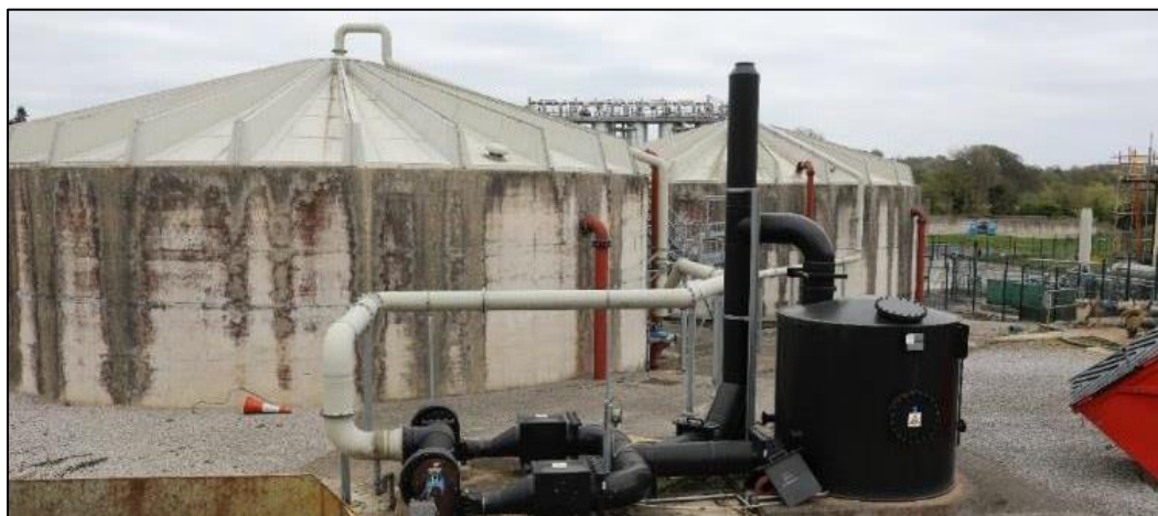
Figure 13. Mixed sludge tanks.
