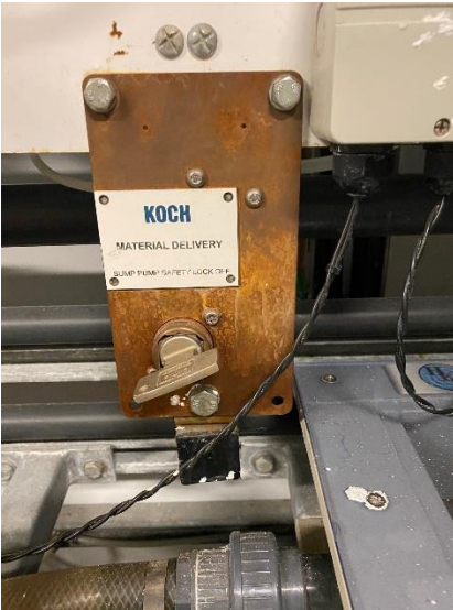
Pump over key box
