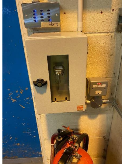
Isolation Valve key box
