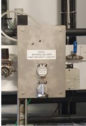
Sump pump lock off
