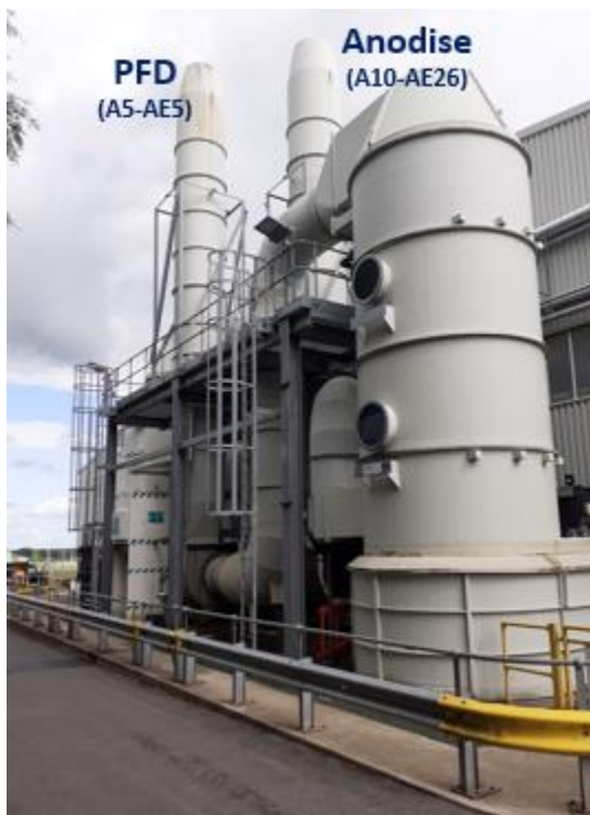
Photograph 2-1: Installed scrubbers at rear of CTF building
