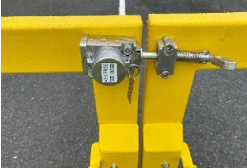
Photograph 4-2: Gate lock fitted with Castell key interlock
