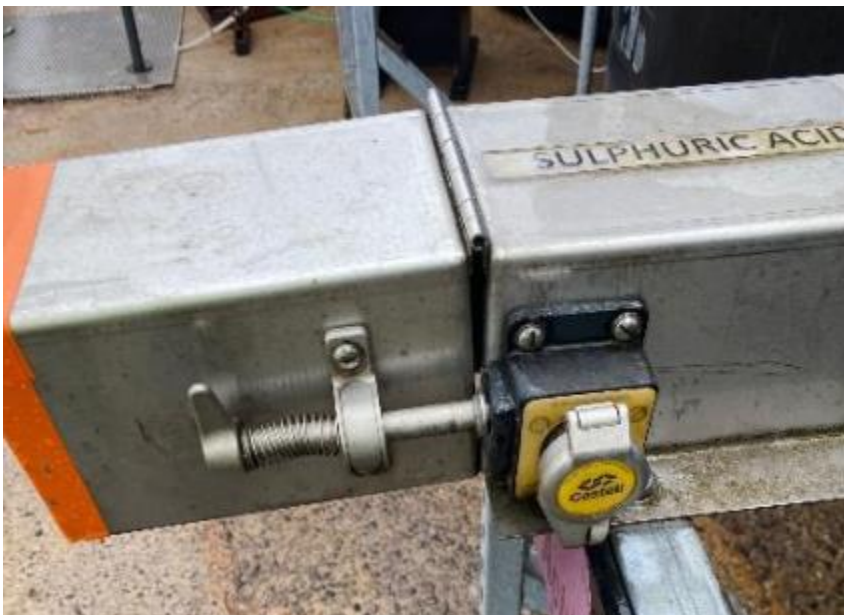
Photograph 4-3: Sulphuric acid pump over Castell key interlock
