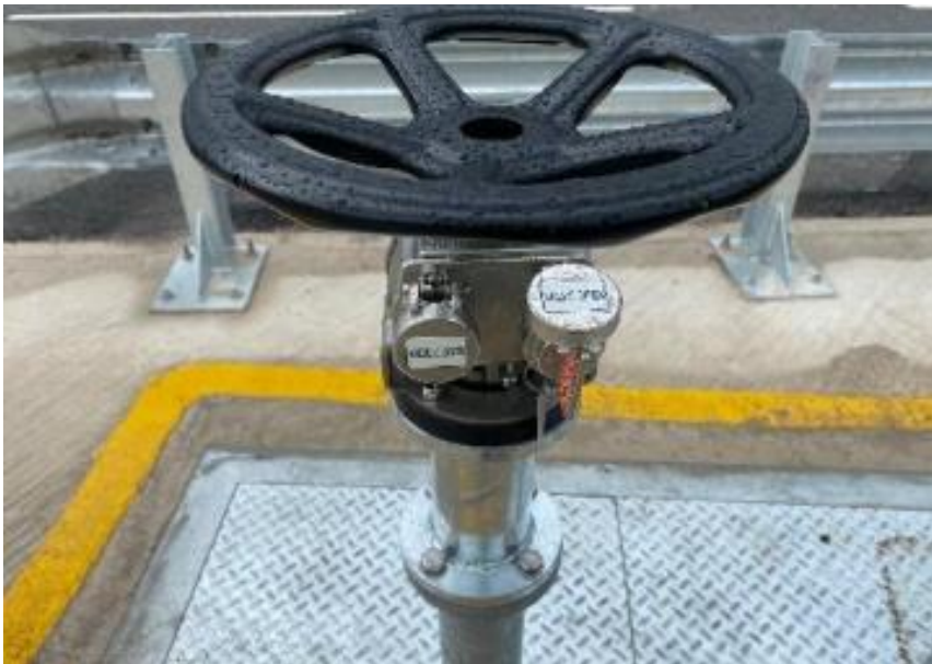
Photograph 4-1: Isolation valve fitted to surface water release (with Castell key interlock)
