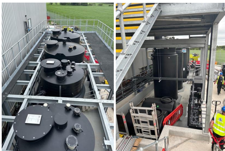
Photograph 3-2: New tanks located within revised secondary containment
