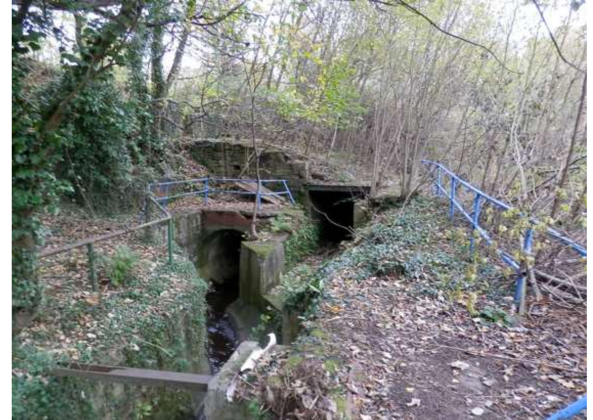
fig 29: connection between the mill race and the River Roddlesworth
