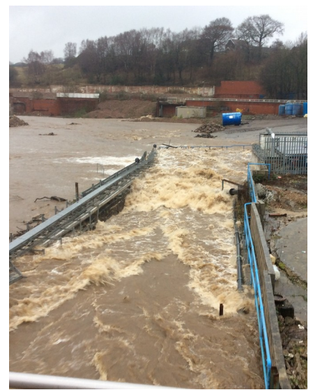
Figure 3.2: Culvert surcharging (Dec, 2012)
