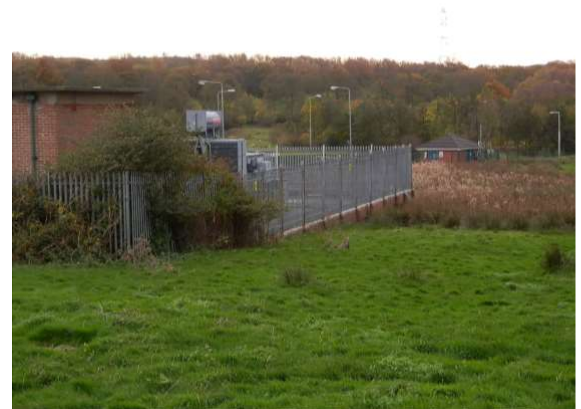
fig 21: view of the sub station from the north
