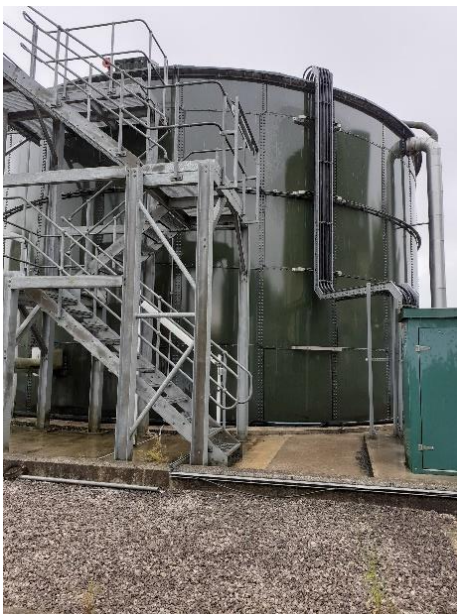
Photo 20: Dewatering Centrate Buffer Tank
