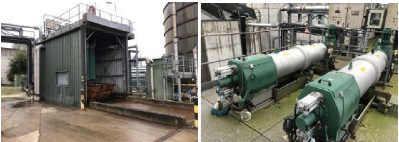
Photos 5 & 6: Sludge Screen Press
