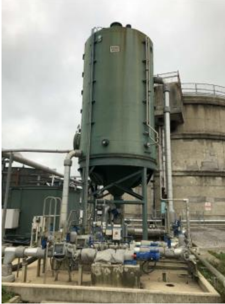
Photo 16: De-gas tank adjacent to Digester
