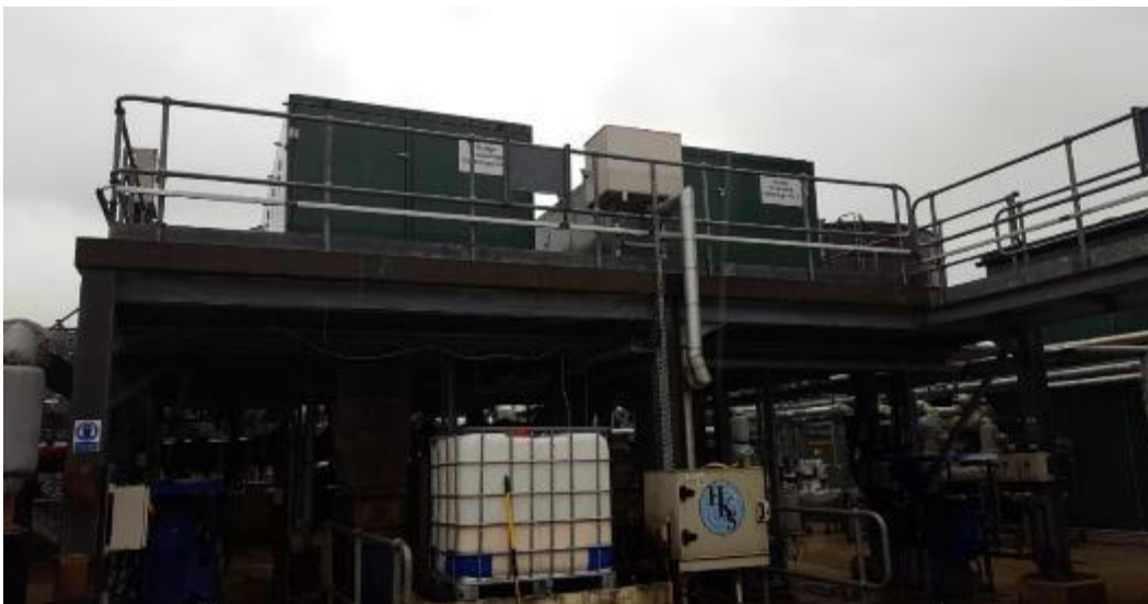
Photo 9: Thickening centrifuges and polyelectrolyte dosing system
