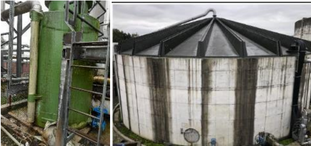
Photos 7 & 8: Buffer storage tank and Screened Sludge Tank
