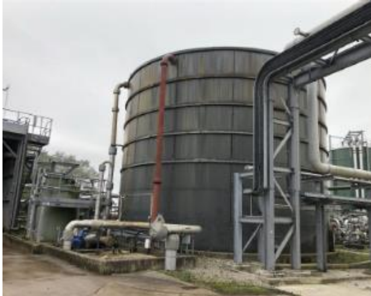
Photo 10: Thickened Sludge Buffer Tank
