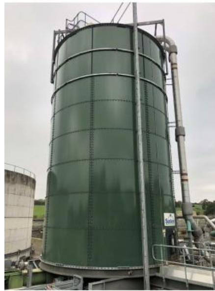
Photo 11: Thickened Sludge Silo
