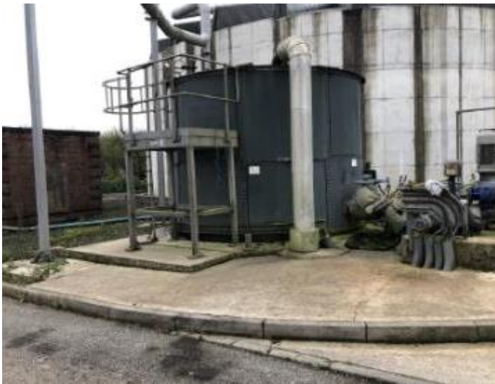
Photo 4: Unscreened Sludge Buffer Tank
