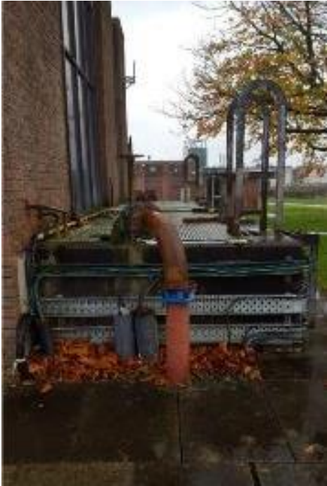
Photo 1: Receiving Wet Well
