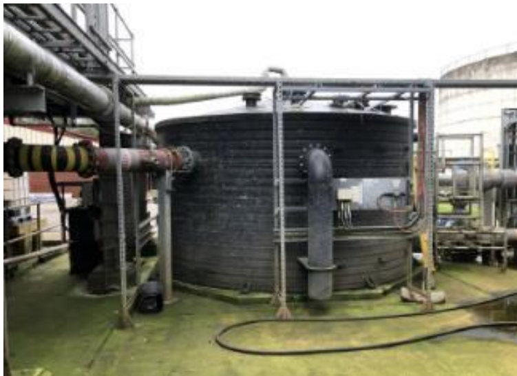
Photo 12: Thickening Centrate Collection Tank
