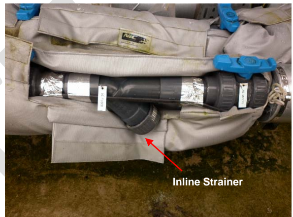
Strainer with lagging removed
