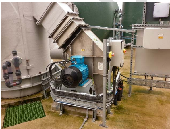
D/S Odour Control Fans
