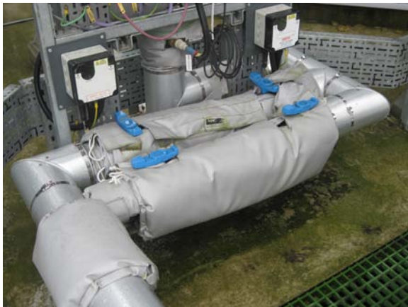
Irrigation Strainers Duty/Standby
