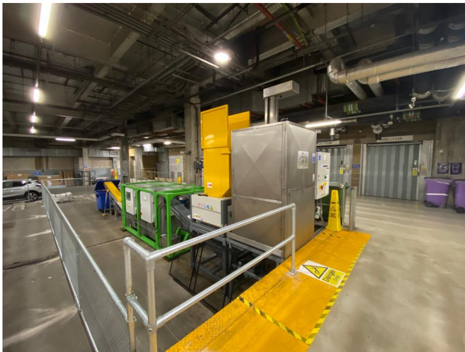
Figure 3 - Advetec Installation at Cribbs Causeway
