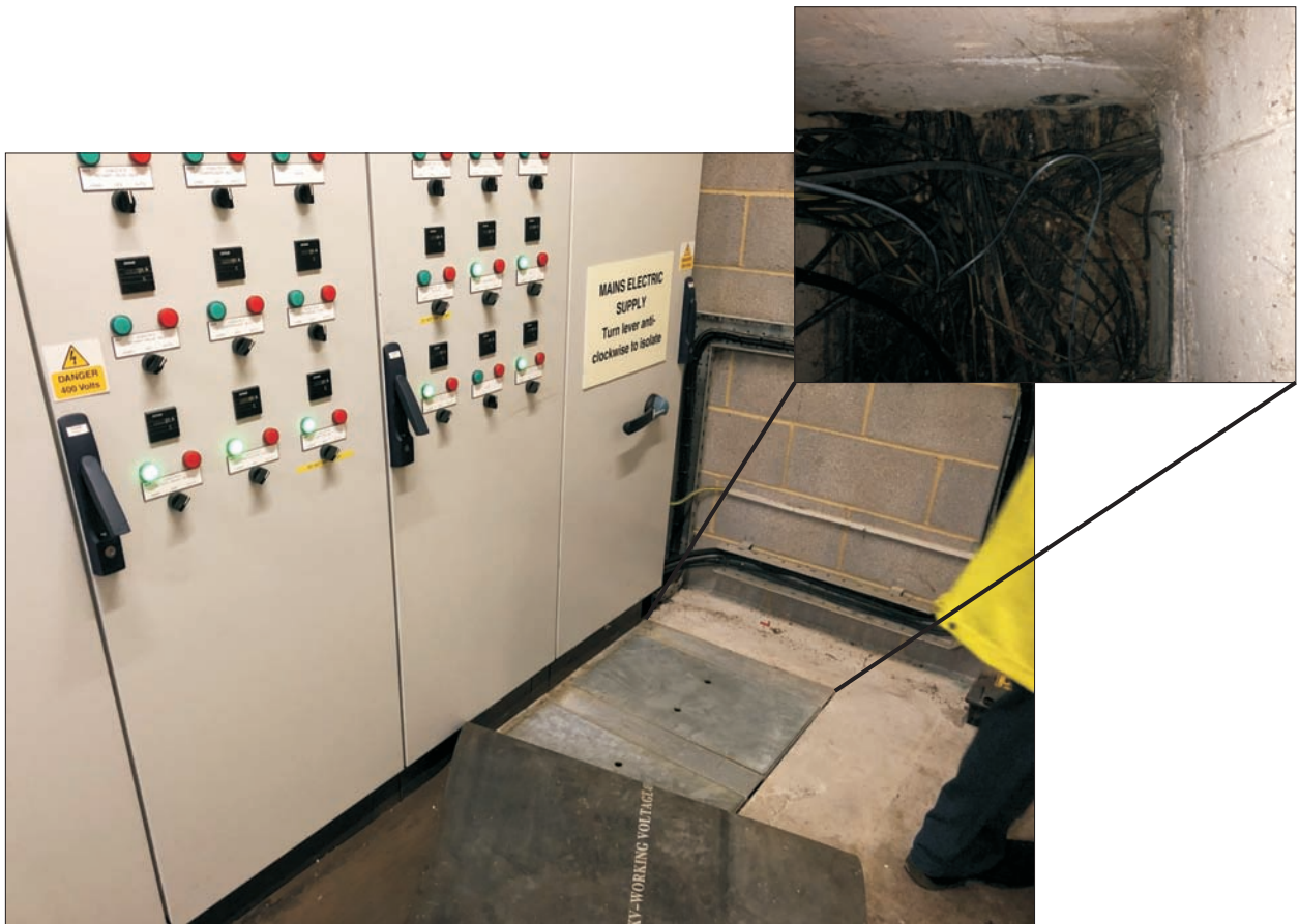
Photo 14. Cables entering control room from AD Plant area (cables linked to Photo 13 area)
