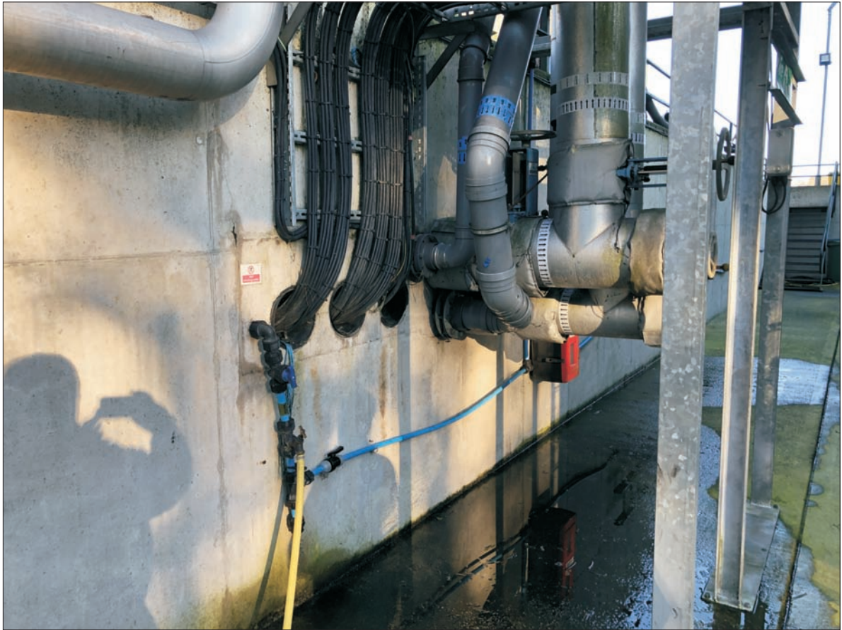
Photo 13. Pipes and cables entering bunded area along western margin of site
