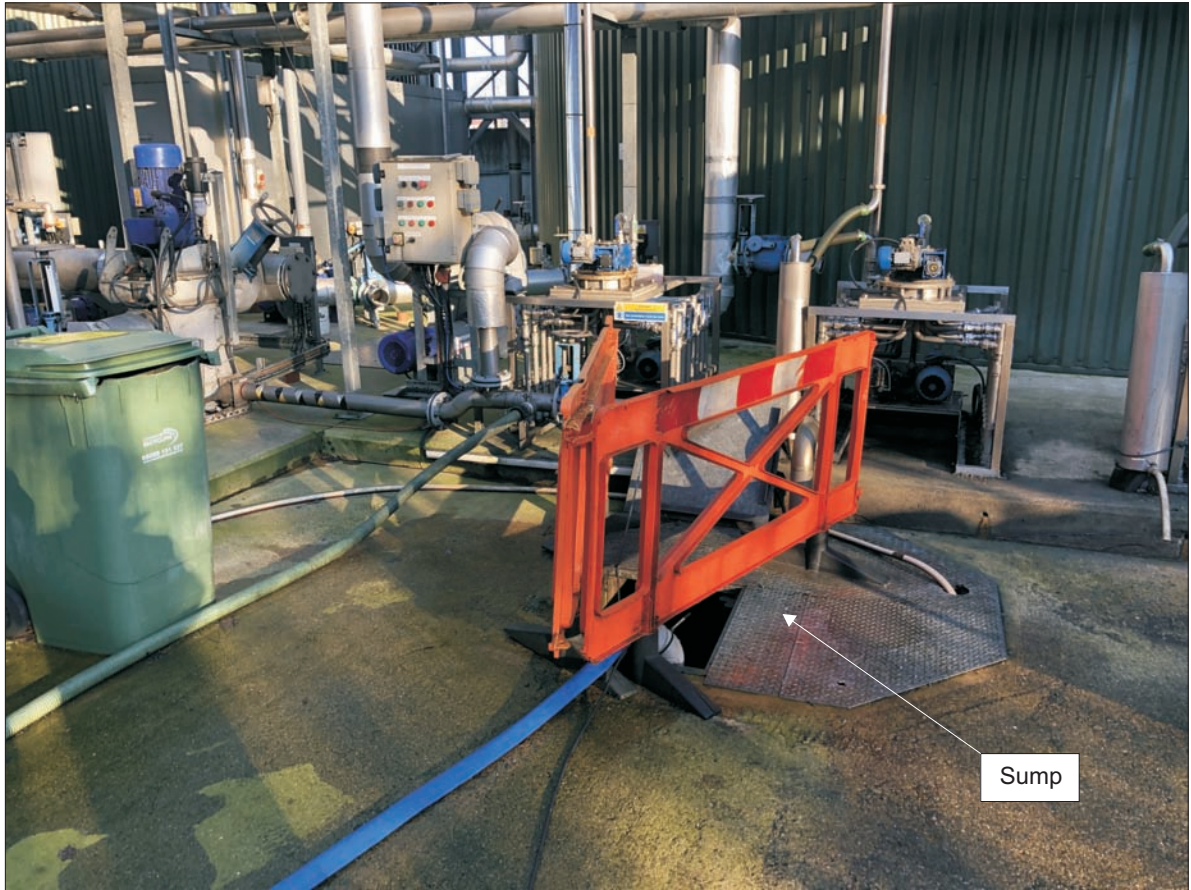
Photo 15. Clean water sump (collection chamber)
