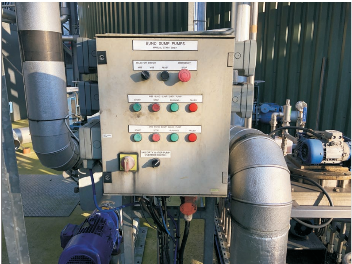
Photo 16. Control panel for pump in clean water sump (manual switch controls)
