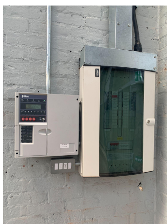
Figure 4 - Fire detection system within the Treatment Building
