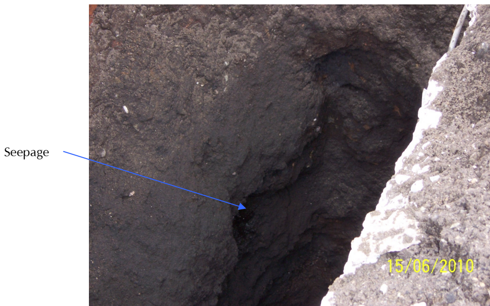
Photograph 4: TPME08 showing seepage into trial pit
