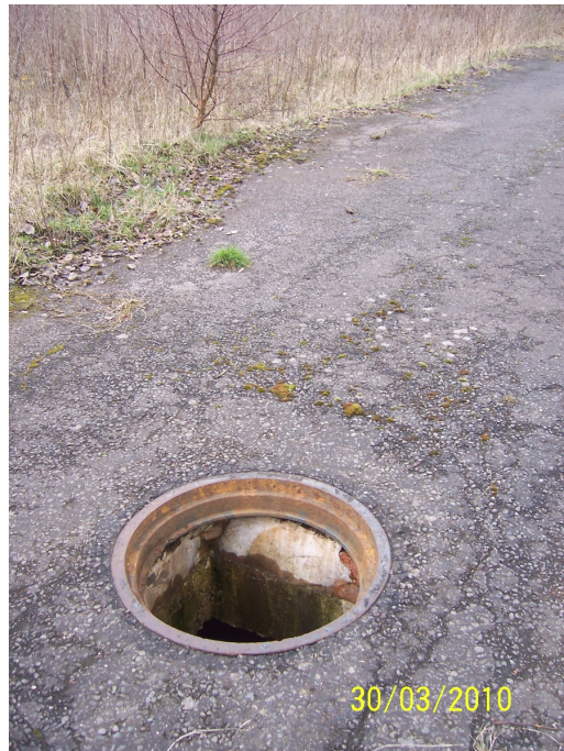
Photograph 6: Missing manhole cover
