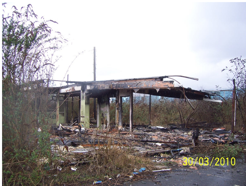
Photograph 10: Burnt out building to the west of the workshops
