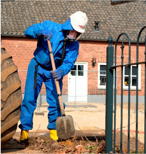
Visual detection of asbestos during remediation | NTP
