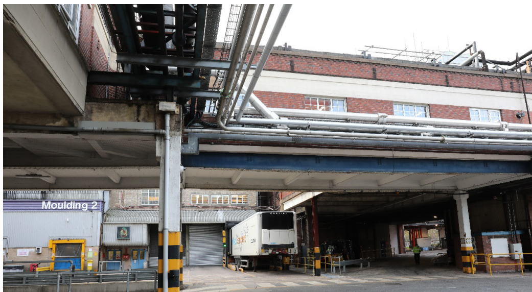
Figure A Stainless steel effluent pipes on pipe bridge
