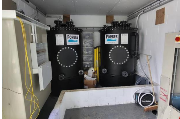
The two hydrogen peroxide storage tanks at the Nent Hags mine water treatment site.
